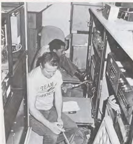
IBM technicians with their backs to the host computer attach cables to the 9020 interfacing switch.
