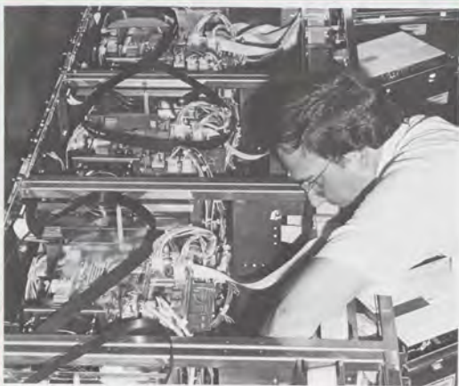
A technician mounts a piece of equipment in a Sperry tape drive rack.
