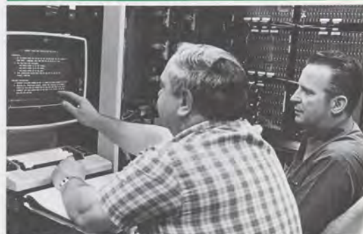
A pair of IBM engineers work at a maintenance processor terminal to evaluate data on the computer system just being installed.
