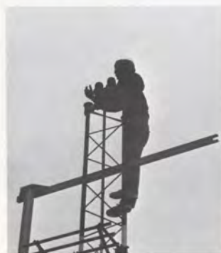
Replacing an obstruction light on the glide slope antenna at Scottsbluff County Airport is electronics technician Joel Myhre.
