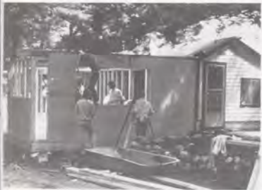
One of the first projects after the purchase of the sheep farm was the addition of a dining hall to the farmhouse, which served as camp headquarters.
