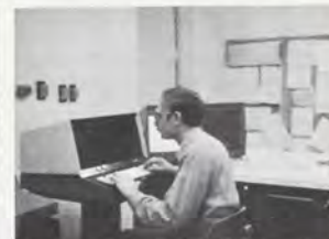
The central control monitoring system computer is used by utility systems technician Anthony Vangeli to check out the TRACON's environmental systems.
