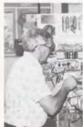
Des Moines navaid technician Einer Jensen maintains one of the 12 VORTACs scattered throughout the sector.
