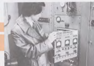
Technician-in-depth Kim Lee checks a component at a remote equipment site.
