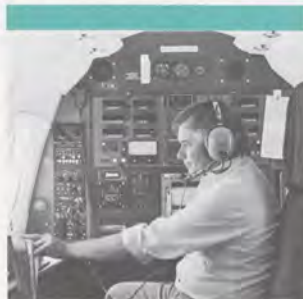
Electronics technician Don Stokes' office during a flight check is a compact, computerized array of avionics at the rear of a Sabreliner flight-inspection plane.
