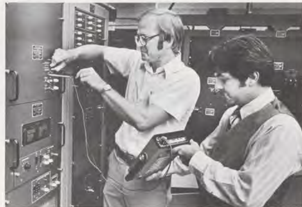
Student Larry Himli plugs into the VORTAC's power supply as instructor Don Torchio demonstrates the use of a multimeter in checking the equipment's internal voltages.
