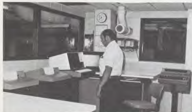
Harvey Buer, assistant chief of the Chicago ARTCC's environmental unit, checks status of the air conditioning system throughout the building with a computerized remote maintenance monitoring system.
