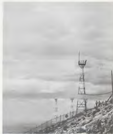
A forest of communications antennas grows atop Mt. Franklin, El Paso, Tex.
