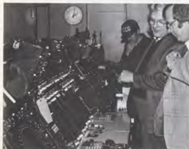
Charles Weaver of the region's Airway Facilities' Communications Staff discusses the trailer-borne TRACON with a telephone company representative.
