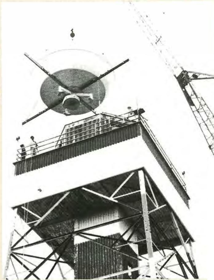
NEW AIRPORT RADAR —Work crews install a new Airport Surface Detection Equipment (ASDE-3) radar at NAFEC/Atlantic City Airport where it's undergoing test and evaluation. The Cardion surveillance radar is expected to increase safety and reduce delays at more than 30 major airports.
