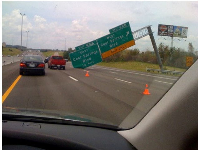
Figure 1.1: Failure of Cantilever Sign Support Structure in Tennessee
