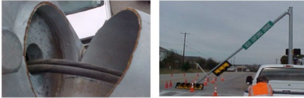
Figure 1.2: Fatigue Failure at Mast Arm Connection of Traffic Signal Source: Florea et al. (2007)
