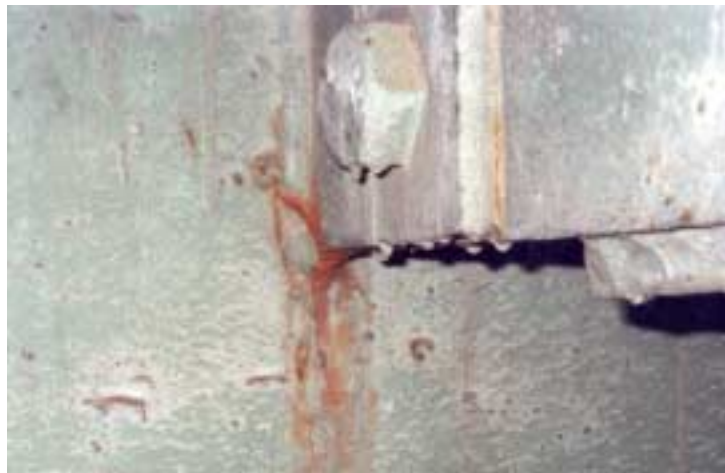
Figure 5.7 Crack C (intermediate crack) on detail side of girder web
