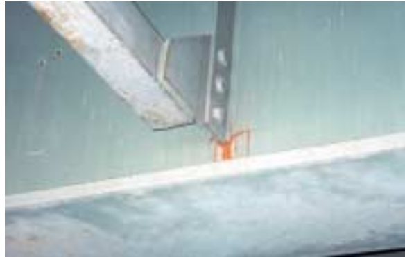
a) Crack A on detail side
