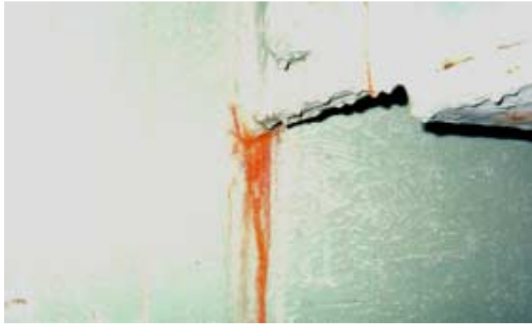
Figure 5.6 Crack B (small crack ) on detail side of girder web
