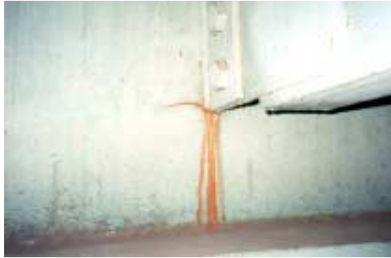
Figure 5.2 Fatigue crack in beam web at cross-frame attachment plate weld
