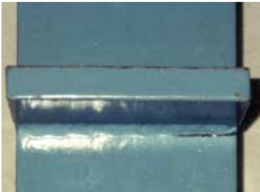
a) 3/8 in. surface crack
