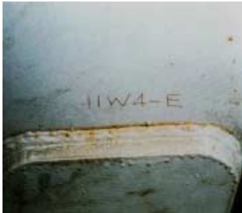
Figure 3.13 Crack in the weld (top) and crack in the member at the weld toe (bottom) (Sung, 1993).
