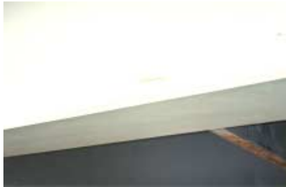
b) Crack A on opposite side
