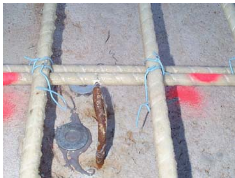
(a) Damaged FRP bar due to repeated rubbing
