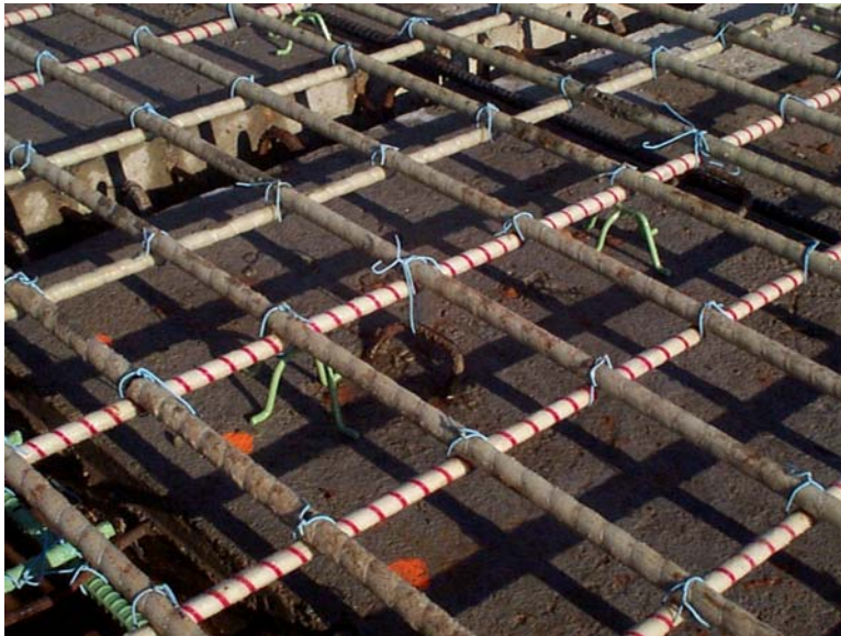
Figure 5.3: Plastic Coated Steel Tie-Wires (Sierrita de la Cruz Creek Bridge, Amarillo, Texas, 2000)
