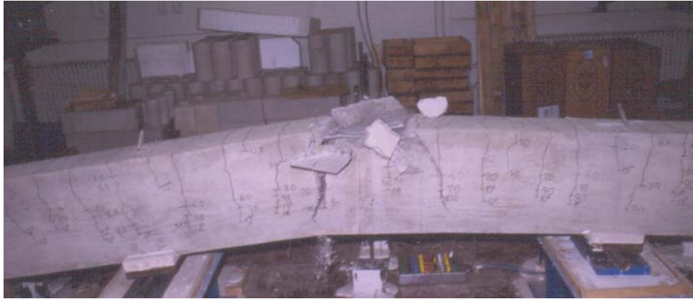
(a.) Wide Angle View of Failure of B-S-2
