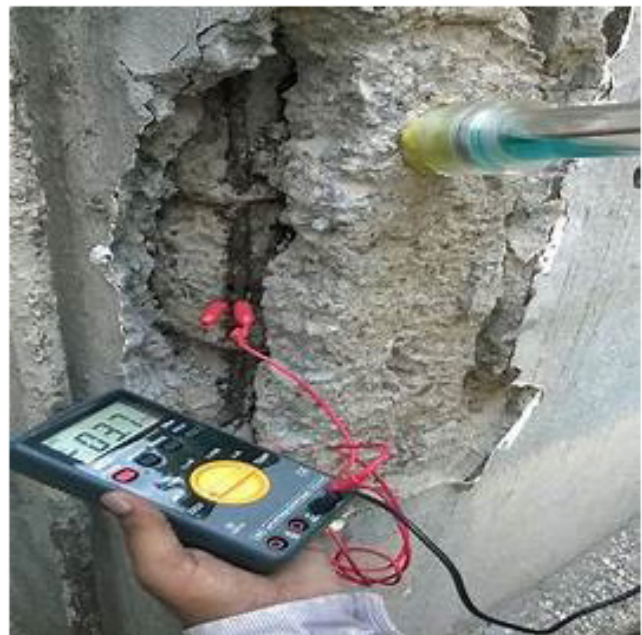
Figure 2.6 HCP Measurement on a Concrete Using a Copper-Copper Sulfate Reference Electrode to Assess Corrosion Activity in Embedded Steel Reinforcement.
