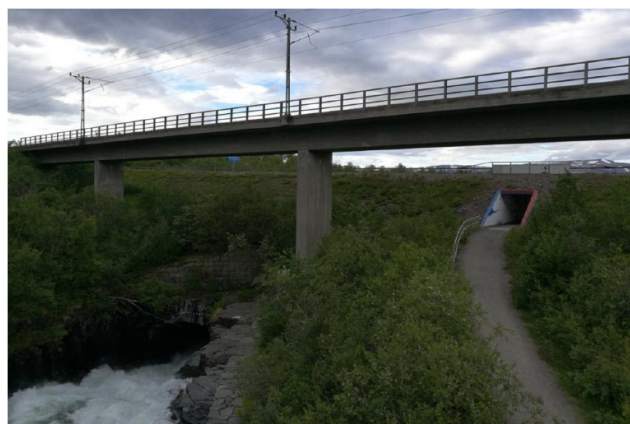
Figure 6.7 The Railway Bridge in Abisko Used for Experiments During the Case Study.
