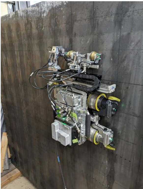
Figure 3.2 Gecko Monarch Climbing Robot Conducting NDT on a Vertical Concrete Wall (Olson, 2025).
