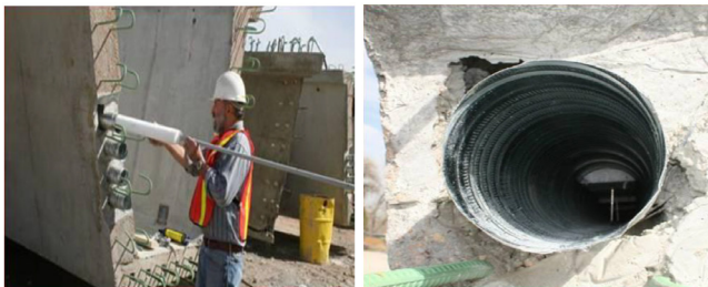
Figure 6.12 Grout Defect Simulation With Styrofoam Voids (Olson, 2025).
