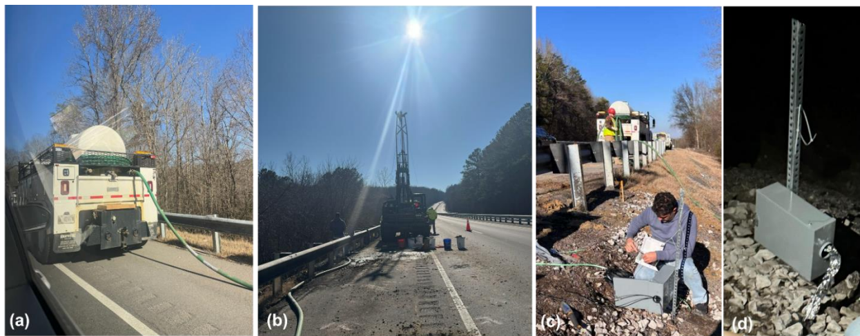
Figure 48. Installation of the in-situ soil moisture monitoring sensor: (a) drilling to prepare the borehole, (b) borehole advancement using the truck-mounted rig, (c) sensor placement and wiring to the data logger enclosure, and (d) final secured instrumentation box and conduit configuration.
