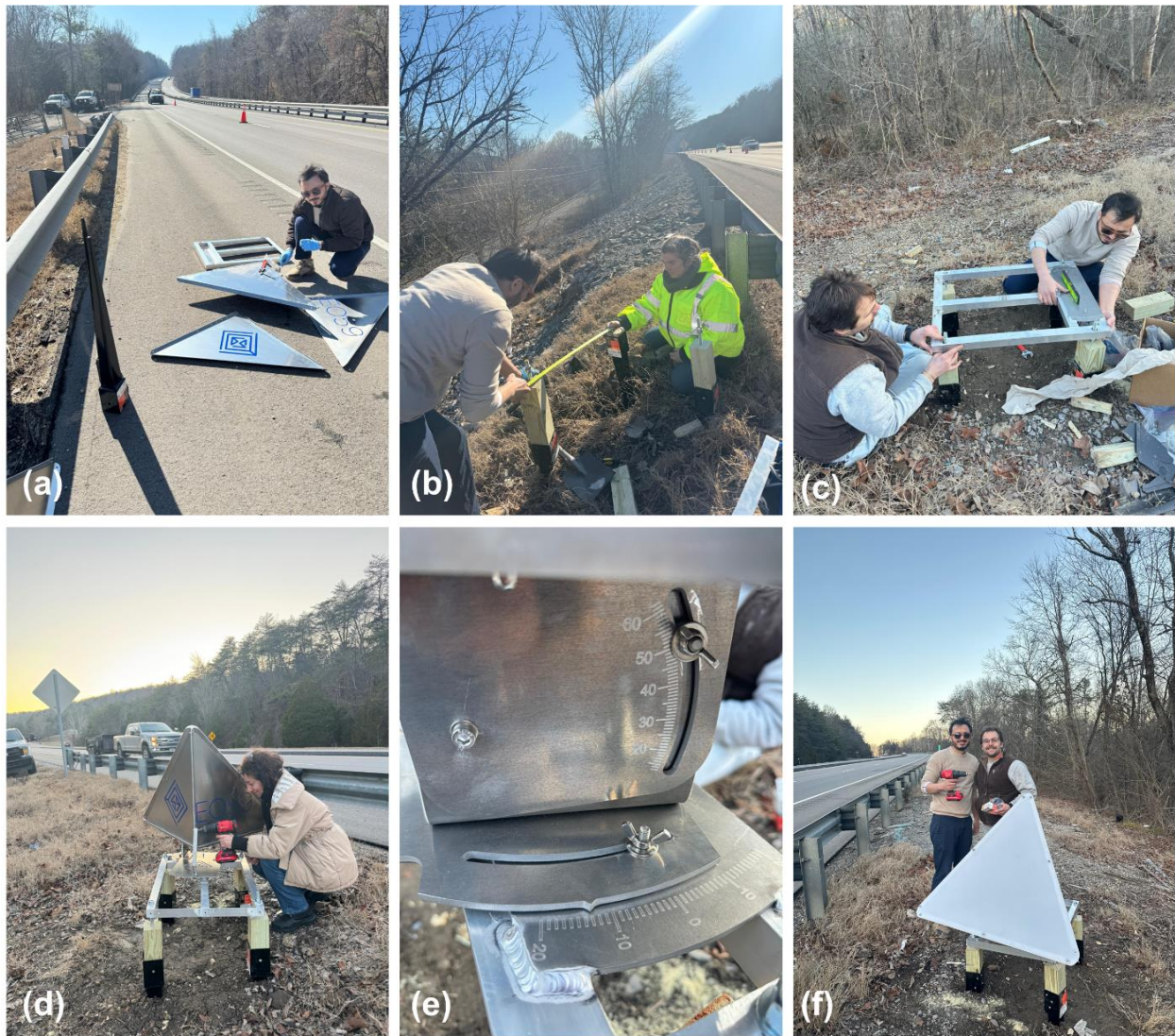
Figure 43. Installation sequence of the corner reflector system: (a) preparation of the reflector plate and base assembly, (b) installation of the timber supports into the ground, (c) adjustment of the base plate position, (d) leveling of the base plate, (e) orientation adjustment toward the satellite line of sight, and (f) final installed configuration.
