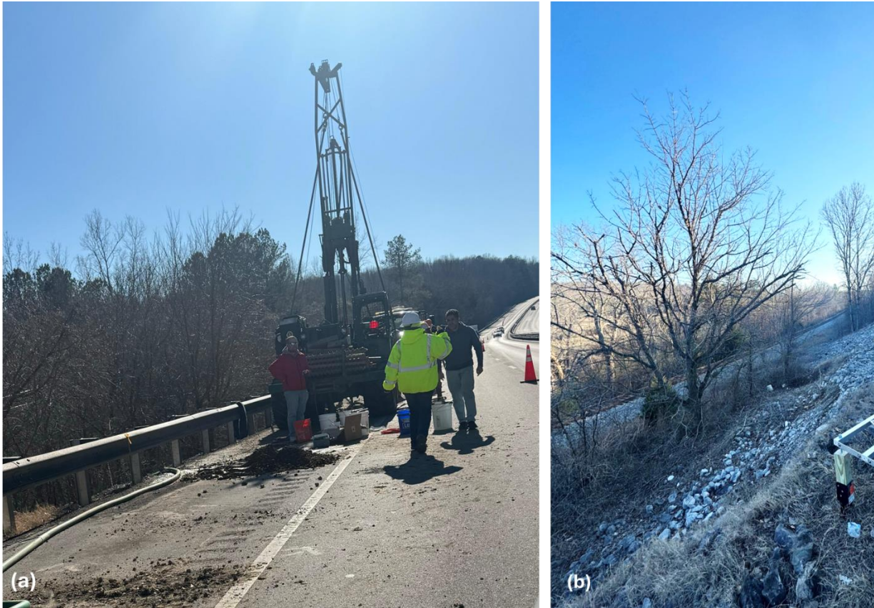
Figure 1. (a) ALDOT drill crews installing subsurface moisture sensors along US-43 near Littleville (Colbert County) to investigate localized ground subsidence. (b) Slope instability area along Littleville Highway (Group 3), selected as the installation location for the second corner reflector.
