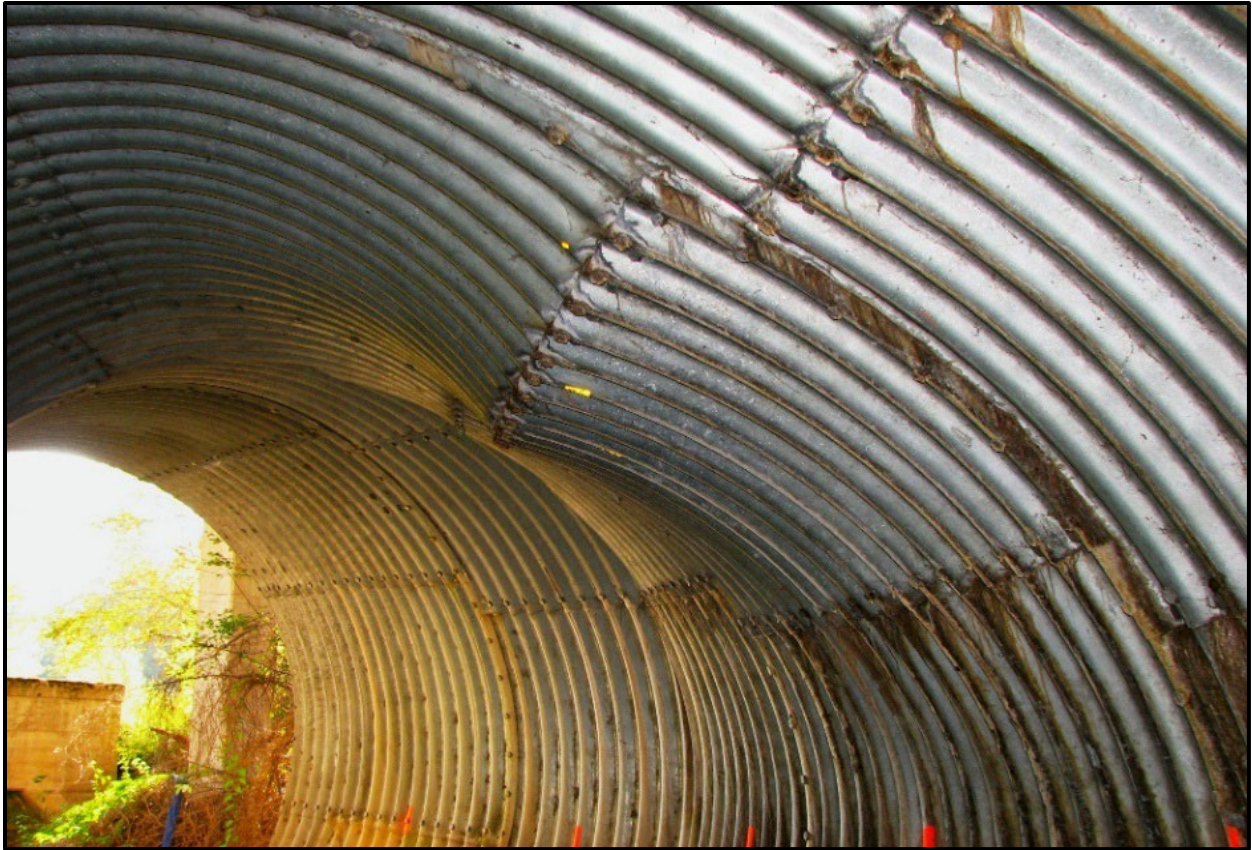
↑ Interior view of extent of steel plate deflection.
