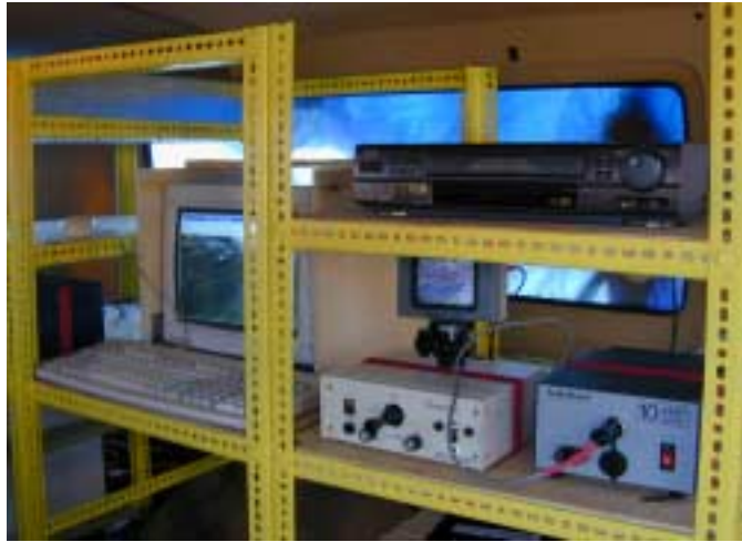
Figure 5.9 Portable Video Detection Control Station
