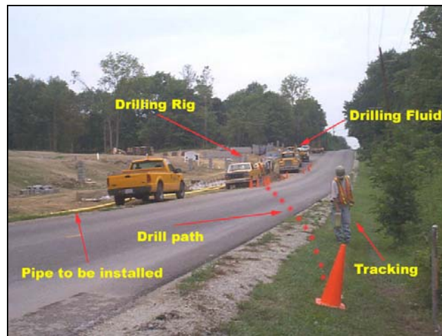
Figure 5.21 Overview of the gas project
