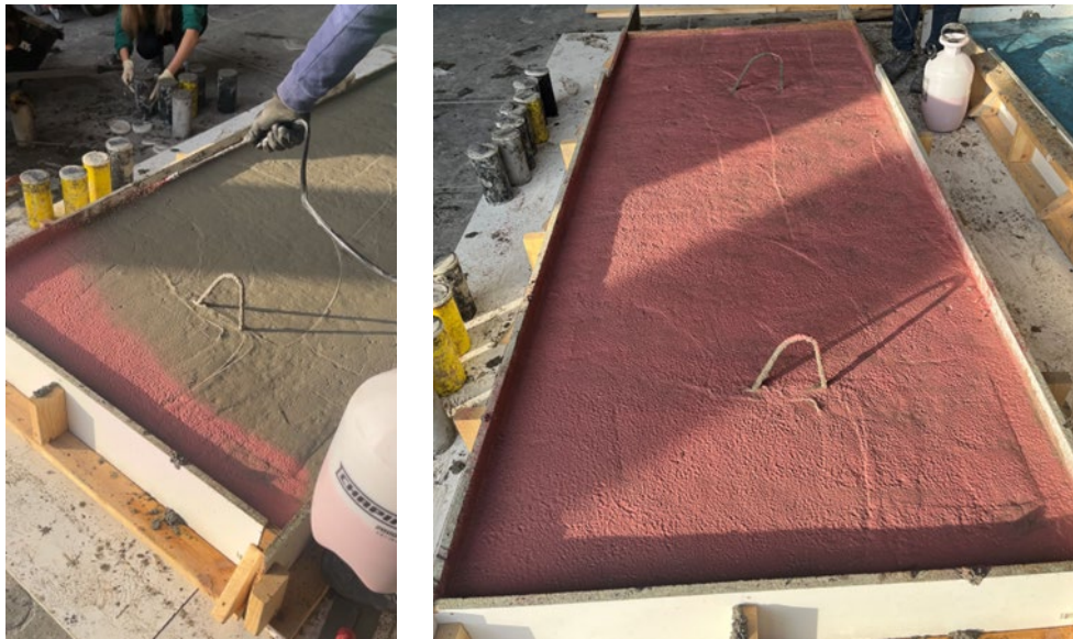
Figure 6.4 Application of Master-Finish XR surface retarder (Pink) from Master Builders on fresh concrete.
