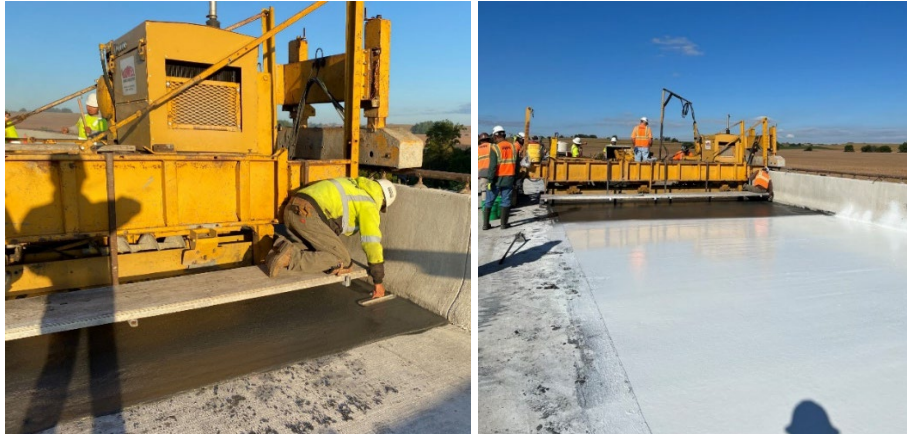
Figure C.8 From left to right: Hand-finishing after paving; Application of white curing compound.
