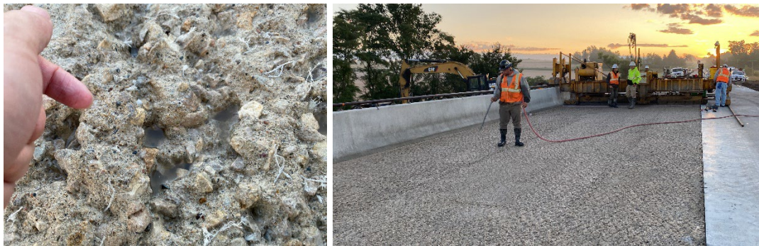
Figure C.2 From left to right: wet surface; removing excess water by air-blowing before the UHPC placement (SSD condition).
