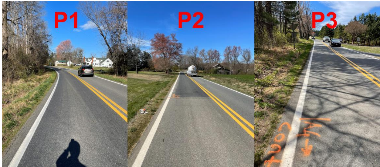
Figure 20. Images of Surface Appearance Approximately 6 Months after Spray-on Rejuvenator Application for Route 640. Treated lane is shown on the left, and untreated lane is shown on the right. P1–P3 denote segments receiving spray-on rejuvenator application.
