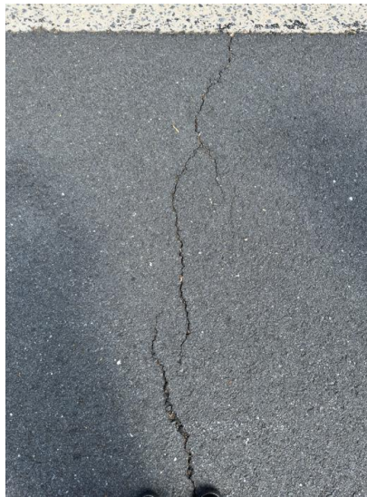
Figure 27. Image of Pavement Surface Condition on Star Flower Drive prior to Treatment
