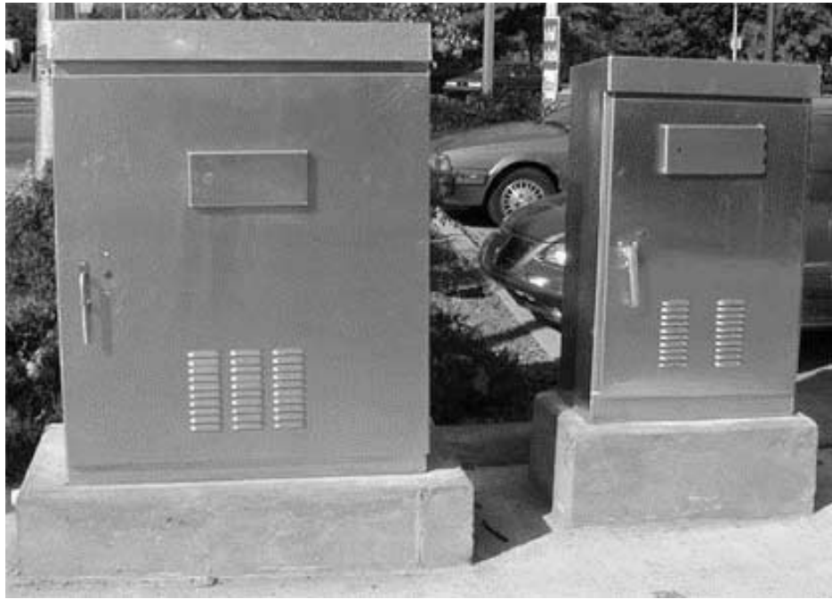
Figure A-3: INDOT and Purdue Cabinets
