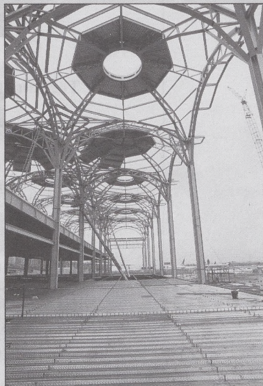
The actual steel structural frame of the new terminal, including modular domed ceiling, is currently under construction.
