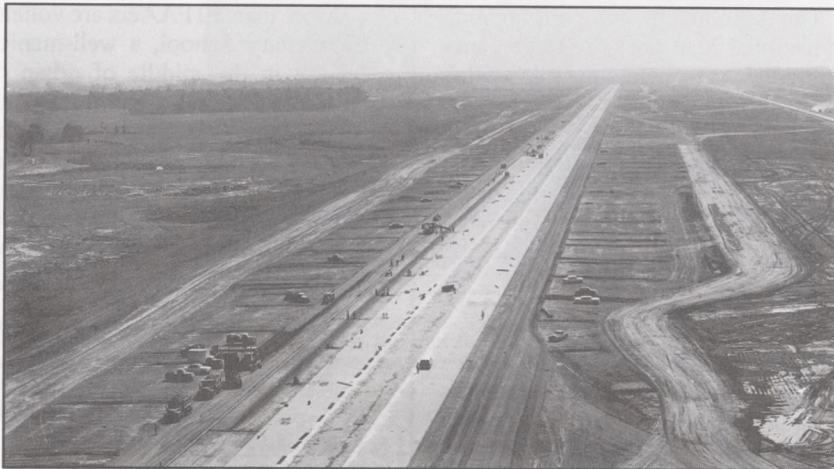
Extending and rebuilding runways is part of DOT's proposal to spur the economy by adding an extra $250 million to airport grants.
