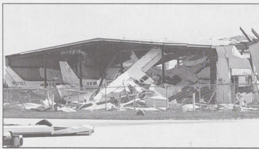
This Tamiami airport hangar was just one of the many casualties of Hurricane Andrew.
