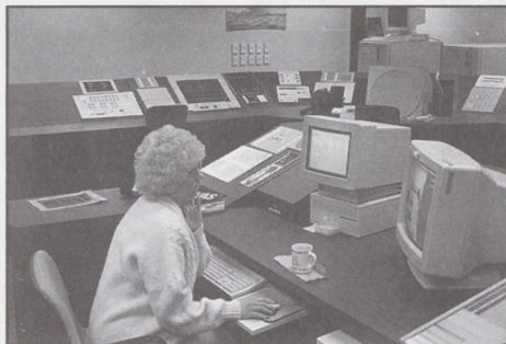
FAA contractor tests one of the many configurations in the new Airway Facilities tower integration laboratory at the Technical Center.
