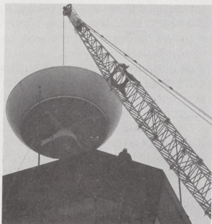
A 300-foot crane raises the ASDE-3 radar above the Pittsburgh airport control tower.
