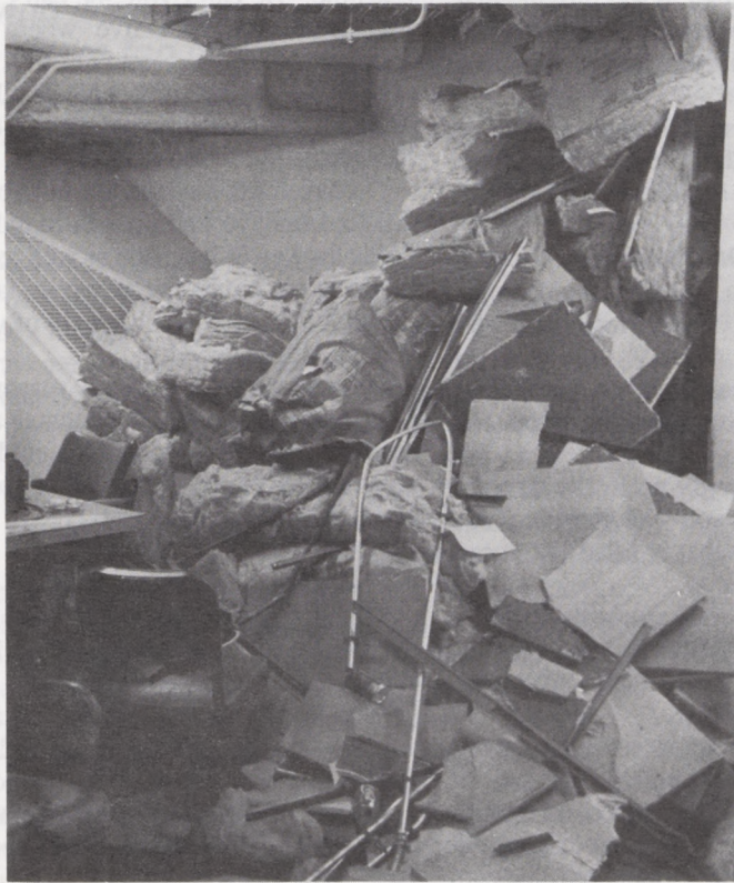
The northern California quake shook the Oakland Air Route Traffic Control Center for about 30 seconds. It knocked panels, ducts and insulation from the ceilings. Despite the severe turbulence, none of the employees abandoned their positions.
