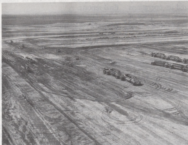
Earth-hauling equipment on the site of the new Denver International Airport moves 100,000 cubic yards of dirt a day. When the site preparation is complete, some 120 million cubic yards of earth will have been moved. The project is running about two months ahead of schedule.
