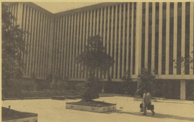
The refurbishing of the courtyard in Nassif Building (DOT) is virtually completed.
