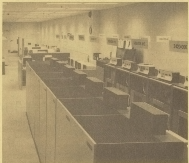
This IBM Host computer, here undergoing tests at the FAA Tech Center, was selected over the system produced by the Sperry Corporation.
