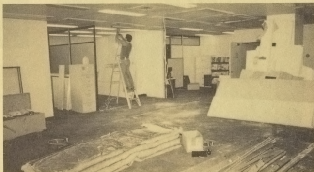
Work goes on as the walls come tumbling down in a third floor office area.
