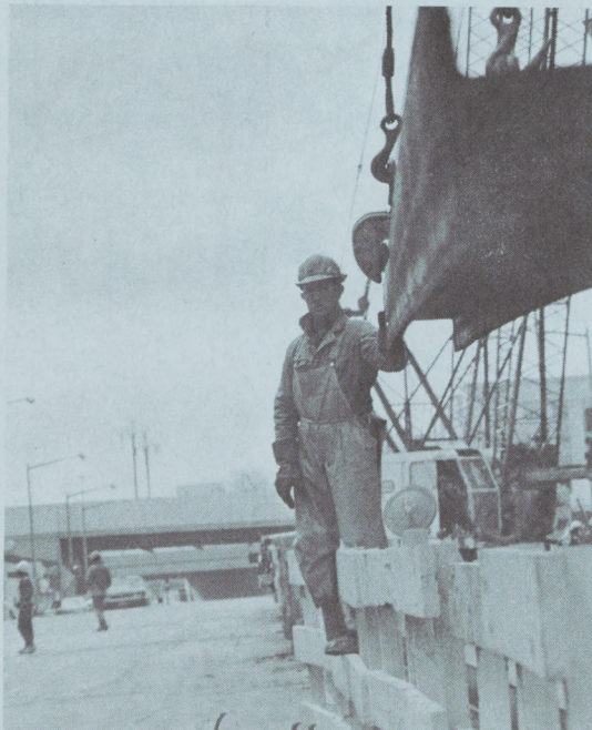
Tons of steel are needed to shore up the street while digging goes on.
