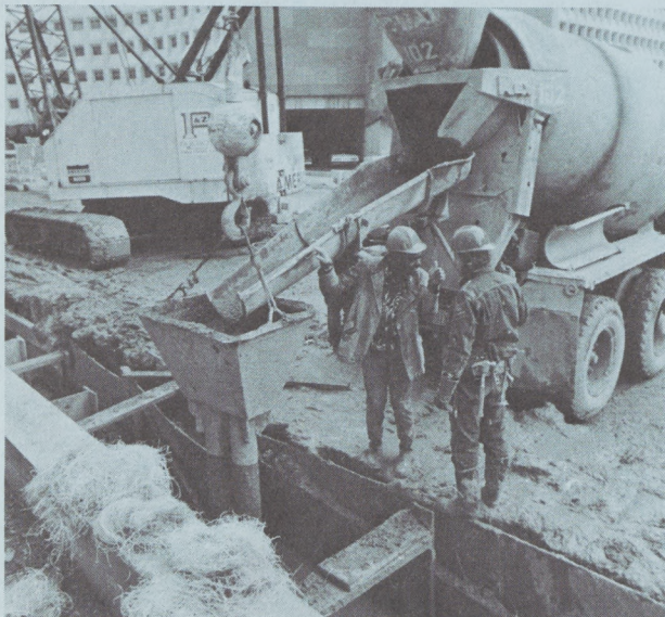
Cement is poured around the soldiers after they're dropped into the holes.
