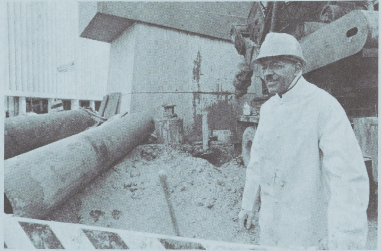
Metro worker stands before smaller bit used to drill holes for under-pinning pipes that will support HUD Building.
