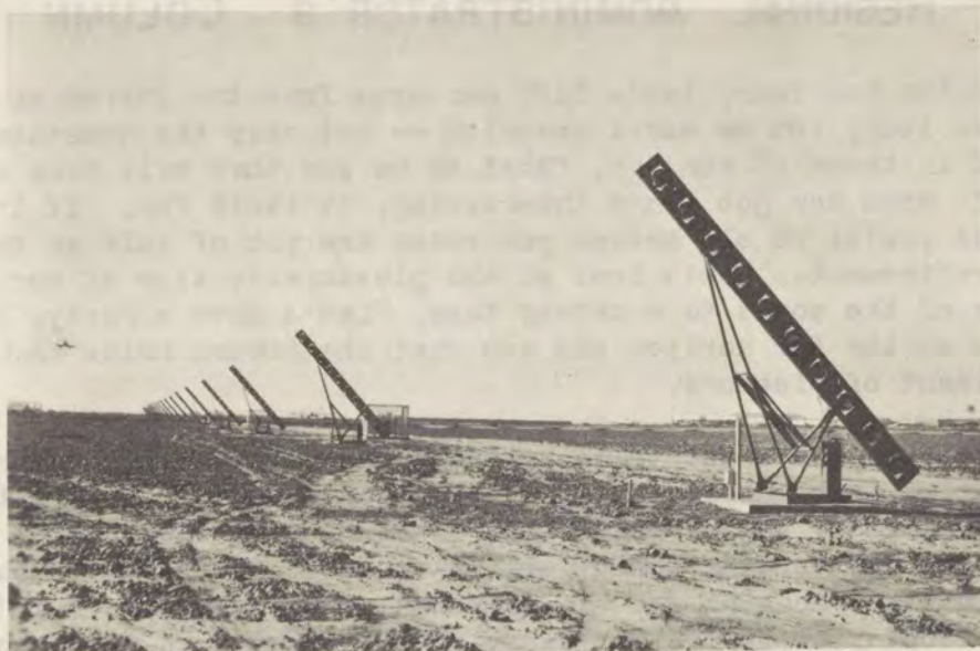
A PORTION OF THE NORTH ROW OF THE SLOPE LINE APPROACH LIGHTS LOOKING TOWARD THE RUNWAY
