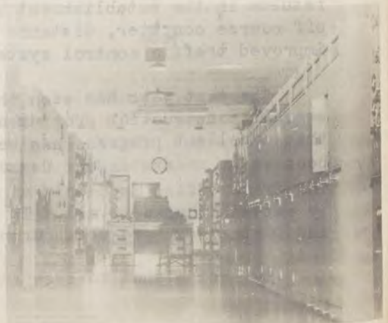
OFACS TRANSMITTER STATION
