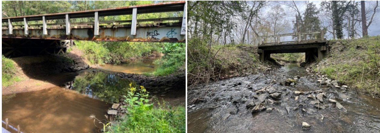
Figure 2. Site 1 Bridge (54.8 feet long, left) and Site 2 Bridge (18 feet long, right) before Construction
