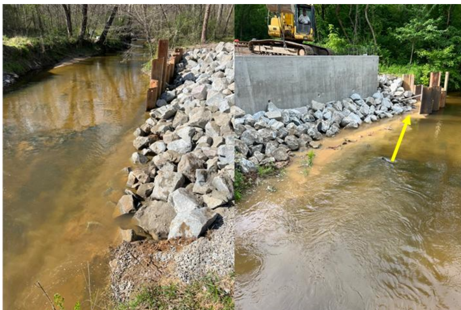
Figure 9. Visible Sediment Plumes during the Removal of the East (left) and West (right) Cofferdams at Site 1. Riprap was placed against the east cofferdam and on top of accumulated sediment, potentially slowing its release and eliminating the need for streambed reprofiling, whereas a space was left between the riprap and west cofferdam (indicated by the yellow arrow).
