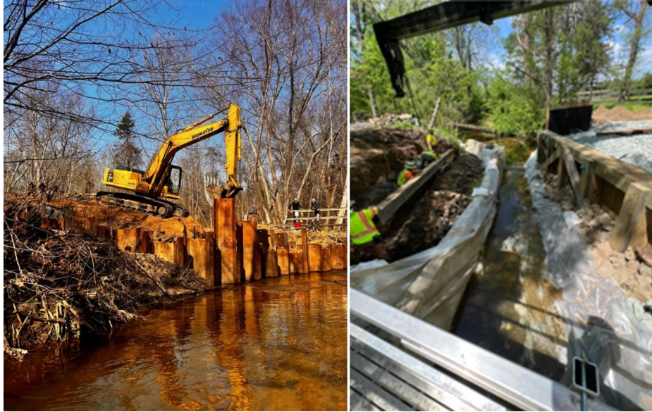
Figure 3. Sheet Pile Cofferdams at Site 1 (left) and Jersey Barrier-Sandbag Cofferdam at Site 2 (right)
