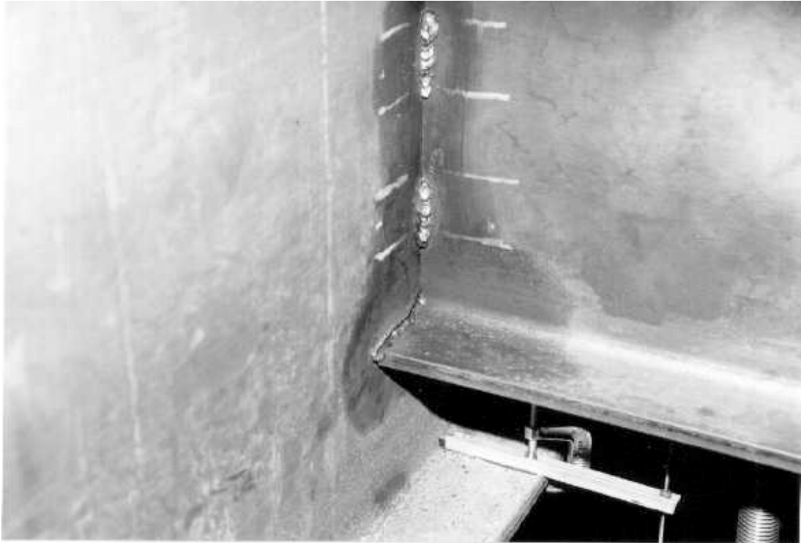
Figure 4.33 Typical fractured bottom weld in nonstaggered diaphragm tests
