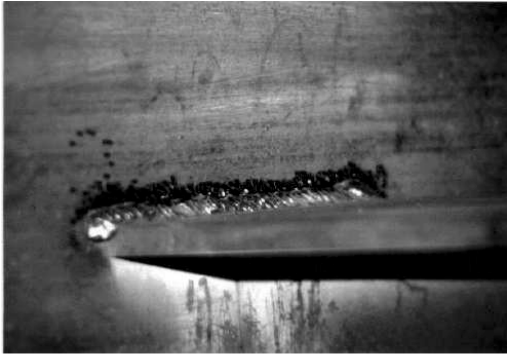
Figure 4.11 Photograph of the peened top flange area
