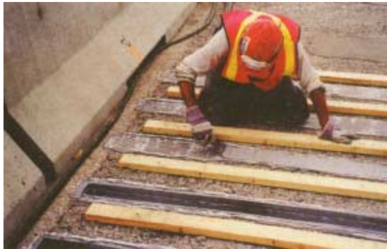
Figure 2.5 FRP strips applied on deck of the Country Hills Boulevard Bridge (Rizkalla and Labossière, 1999)
