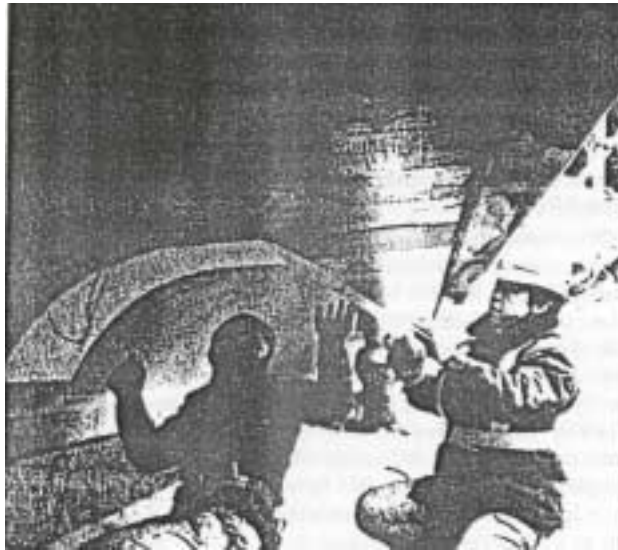
Figure 2.2. Installation of FRP sheets on the soffit of the cantilevered slab of Hata Bridge (Nanni, 1995)
