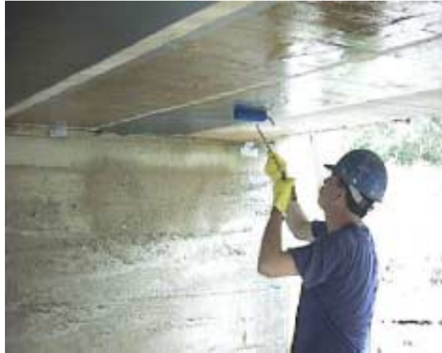
Figure 2.8. Application of the adhesive to the underside of the deck (Mayo et al., 2000)
