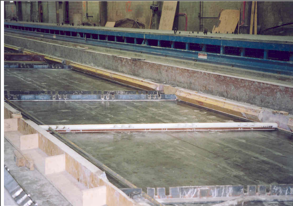
Fig. 68. Plastic rod over fiber board at hinge section during fabrication of NU-Deck panels for the Skyline Bridge (Versace, 2003)
