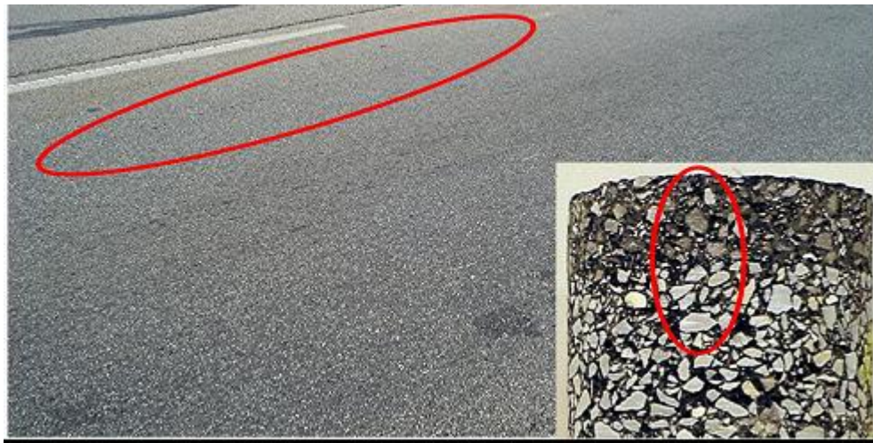
Figure 1: Surface cracked major interstate highway (I-65 North) in Indiana.
