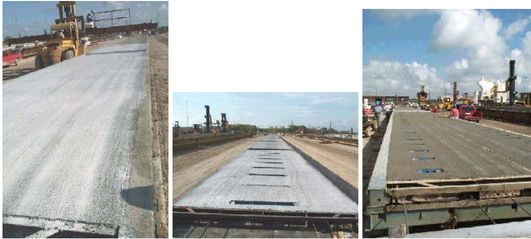
Figure 4.18. Finished set of base panel, central panel, joint panel (from left to right) in the casting bed
