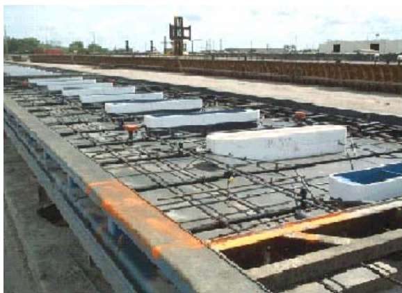
Figure 4.10. "Boxes/inserts" are placed for preparing the stressing pockets of central stressing panel mold
