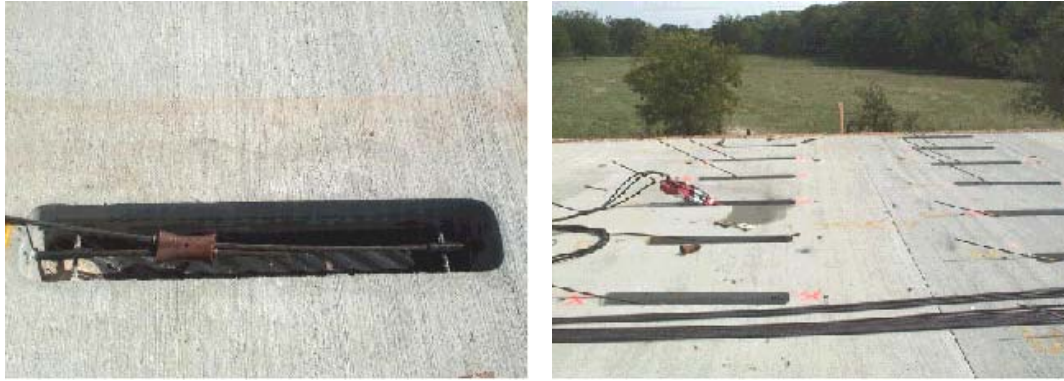
Figure 4.30 Strands from each end of the slab are coupled together (left) and tensioned in the central stressing pockets (right)
