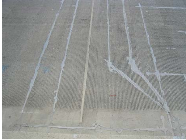
Figure 4-6 Concrete Cracks in CDS deck system
