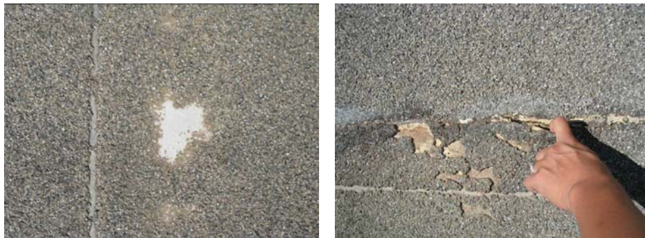
Figure 4-4 Debonding of the wearing surface
