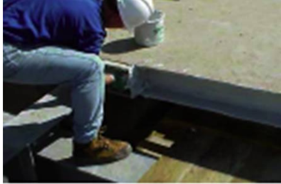
Figure 2-14 Liquid Primer and Epoxy Paste to being applied the Field Joint (Source: MMC 2003)
