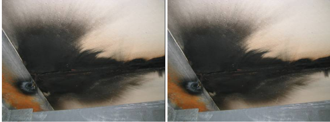
Figure 4-13 Fire damage found in the bottom of panels
