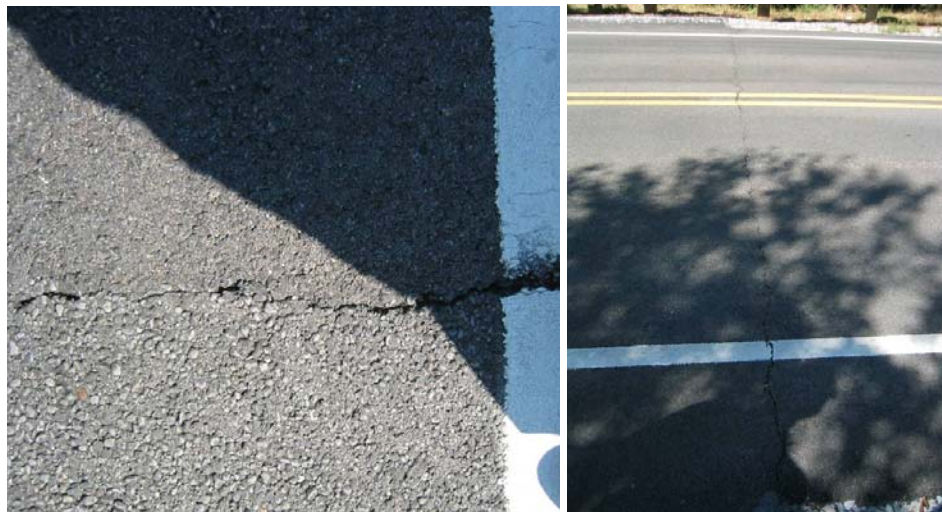
Figure 4-19 De-bonding, and cracking of Wearing surface
