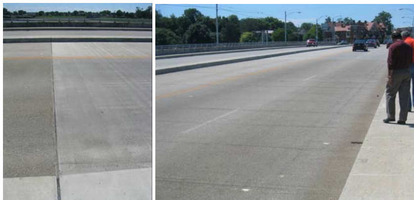
Figure 4- 5 Wearing surface cracking at a deck joint
