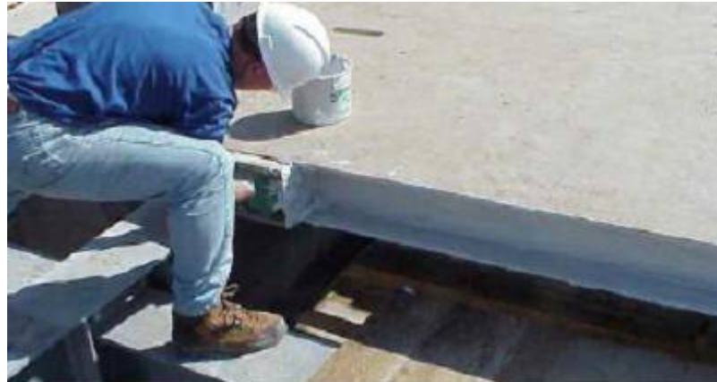
Figure 5-9 Liquid primer and epoxy paste applied to field joints (Source: Busel and Lockwood 2000)
