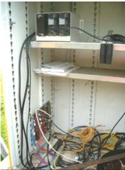
b) Loop output in cabinet 1
