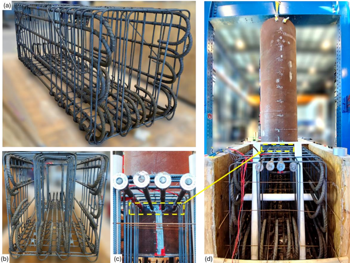
Figure 3-2 Photos of Bent Cap Rebar Cage: (a) Isometric View, (b) Face View, (c) Close-up of Headed Rebars Crossing the Pipe Pile, and (d) Bent Cap Rebar Cage with Pipe Pile
