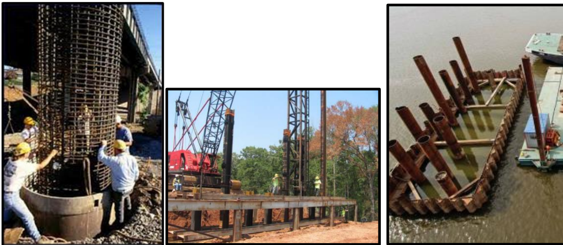
Figure 1-1 (a) RC drilled shaft Steel (Brown et al., 2010); (b) HP piles (Voyiadjis et al., 2016); (c) Large diameter steel piles (Brown et al., 2015)
