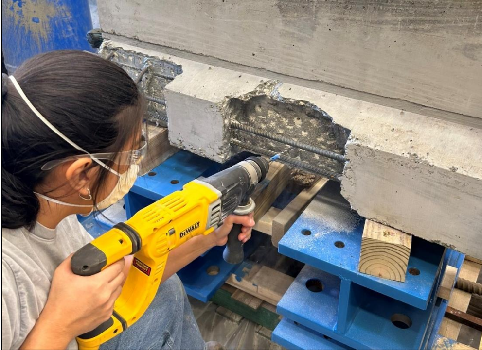
Figure 33. Photo. Practice hammer-drilling pilot holes for concrete anchors between closely spaced reinforcement.
