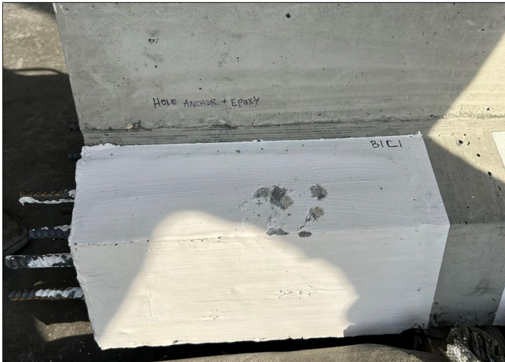
Figure 41. Photo. Minimal surface chipping after sledgehammer impact. The sledgehammer did not crack or dislodge the patch.
