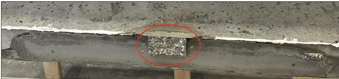
Figure 9. Imperfection due to chimney opening.
