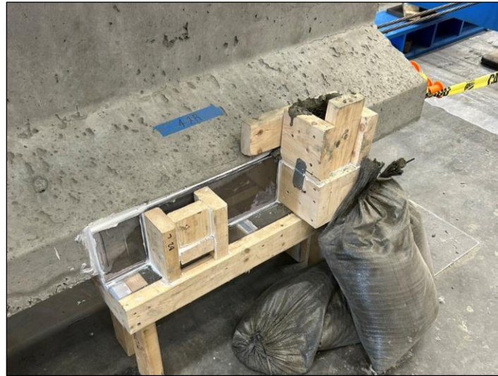
Figure 63. Photo. Sandbags keeping the formwork stable after SCC replacement of the repair void.
