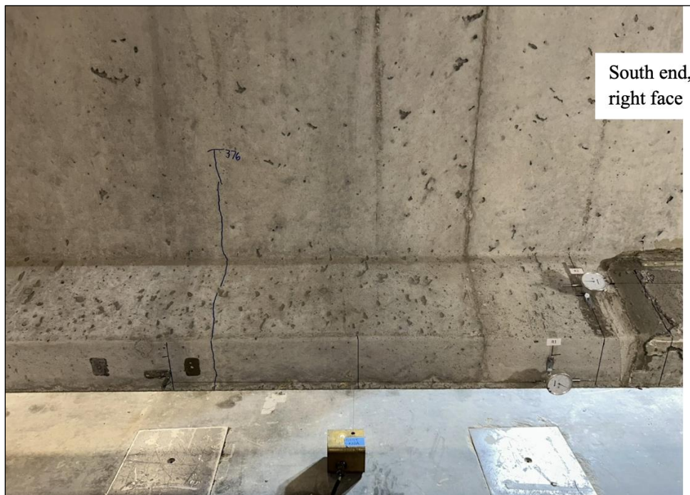
Figure 148. Photo. Test 3.2.S (repair 3.2RBF) flexural cracks toward the midspan, to the left of repair 3.2RBF at 376 kip (right face of girder pictured).
