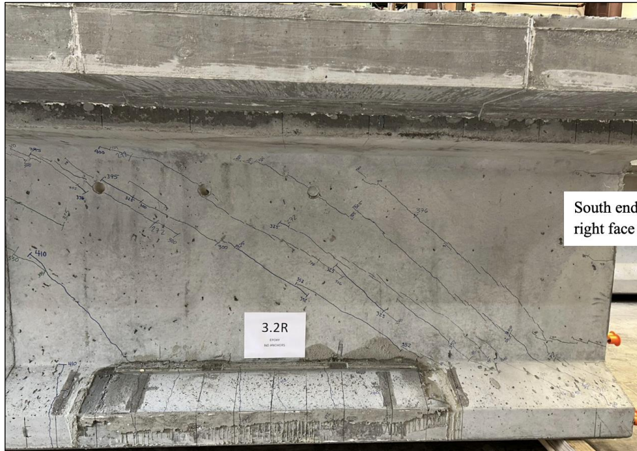
Figure 152. Photo. Test 3.2.S (repair 3.2RBF) final shear cracks on repaired face of the girder at 410 kip (right face of girder pictured).
