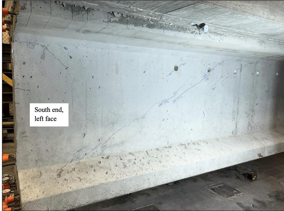
Figure 147. Photo. Test 3.2.S (repair 3.2RBF) initial shear cracks on nonrepaired, original girder face at 272 kip (left face of girder pictured).
