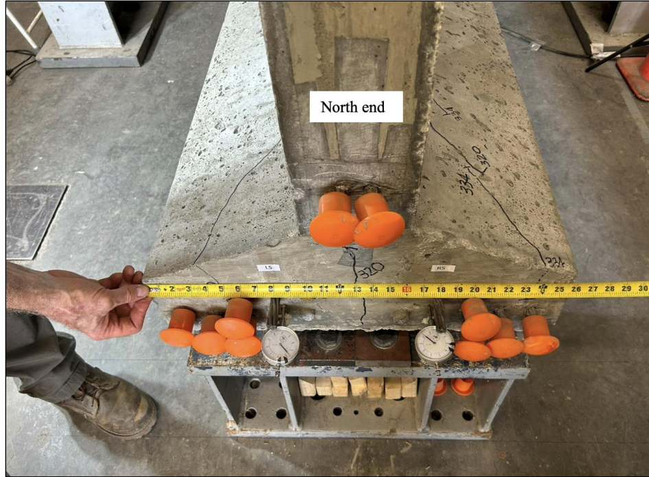
Figure 111. Photo. Test 2.1.S (repair 2.1RTF, 2.1LTF) north end cross-section cracks extending past center of bearing, prompting strand slip failure.
