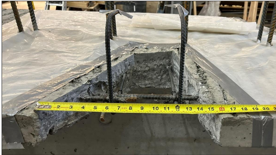
Figure 1. Top flange nonconformity not located at the end of the girder.
