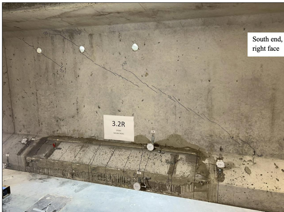
Figure 146. Photo. Test 3.2.S (repair 3.2RBF) initial shear cracks not going through repair 3.2RBF at 272 kip (right face of girder pictured).
