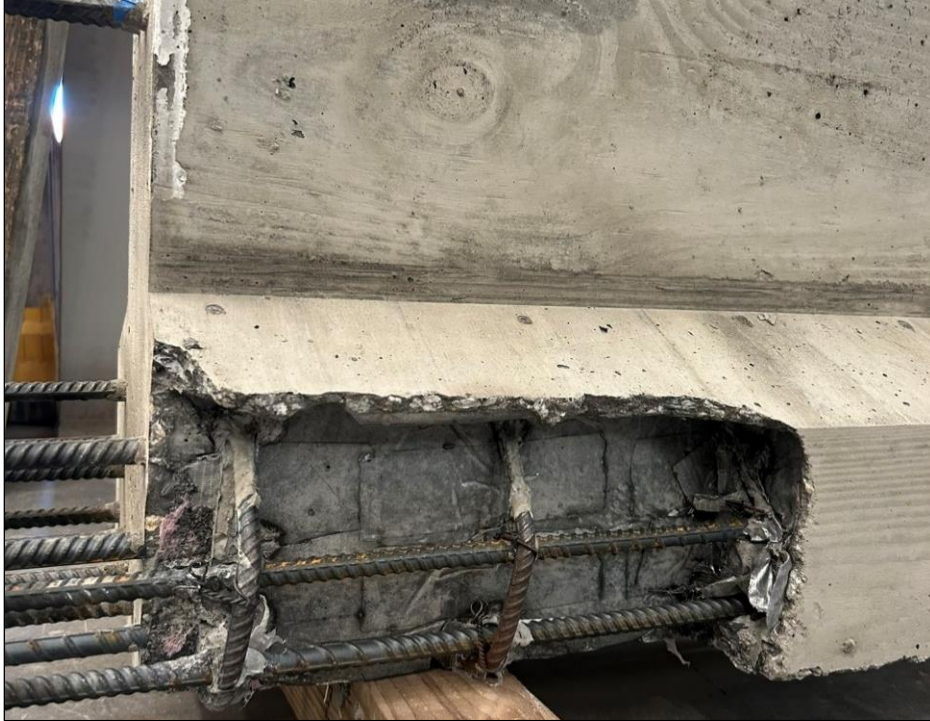
Figure 31. Photo. Mini girder nonconformance representing conditions comparable to repair 3.1RTF.
