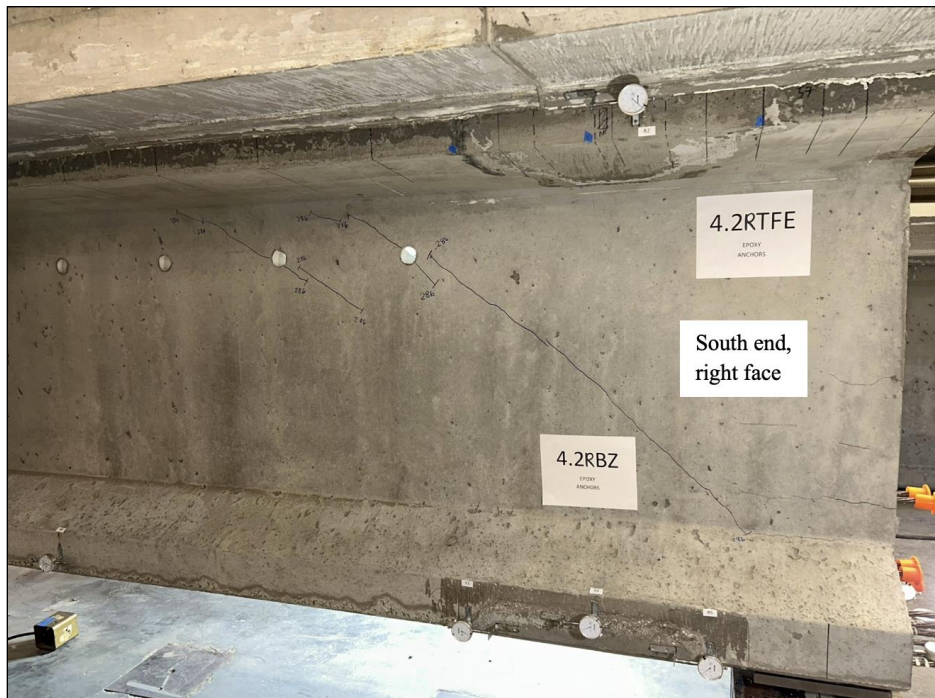
Figure 175. Photo. Test 4.2.S (repair 4.2RBZ, 4.2RTFE, 4.2RTF, 4.2LTF) initial shear cracks on repaired face at 286 kip (right face of girder pictured).
