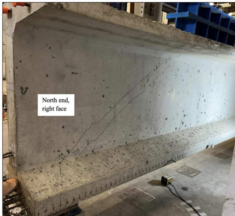
Figure 83. Photo. Test 1.1.S (repair 1.1LBZ) initial shear cracks on the original, nonrepaired girder side (right face of girder pictured). Note that the diagonal cracks orient to a location over the center of the end support.
