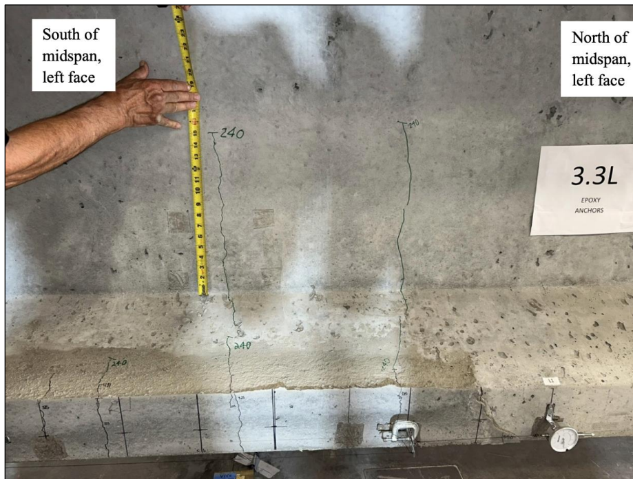
Figure 158. Photo. Test 3.3.F (repair 3.3RBF, 3.3LBF) initial flexural cracks extending 15 in. from the top of the bulb at 240 kip (left face of girder pictured).
