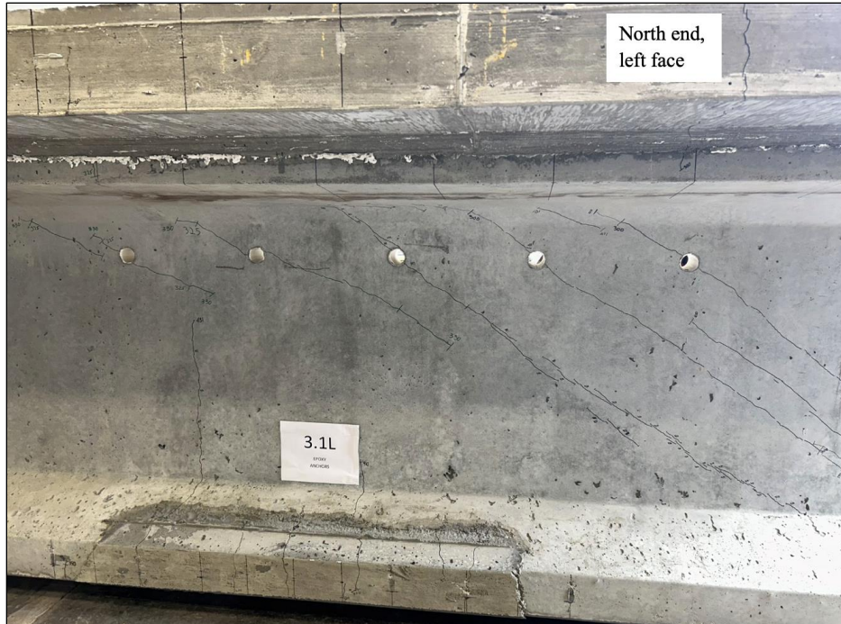
Figure 142. Photo. Test 3.1.S (repair 3.1RBF, 3.1LBF) final crack pattern at 431 kip (left face of girder pictured).
