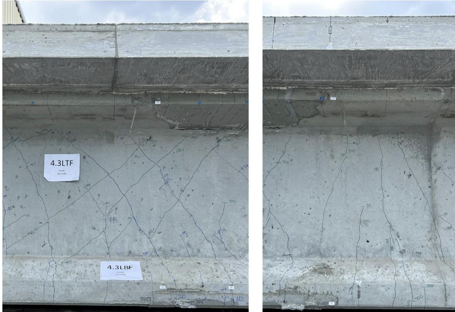
Figure 191. Photo. Test 4.3.F (repair 4.3LBF, 4.3LTF) final overall crack pattern on the top and bottom flange repaired girder face after the final load of 331 kip (left face of girder pictured).
