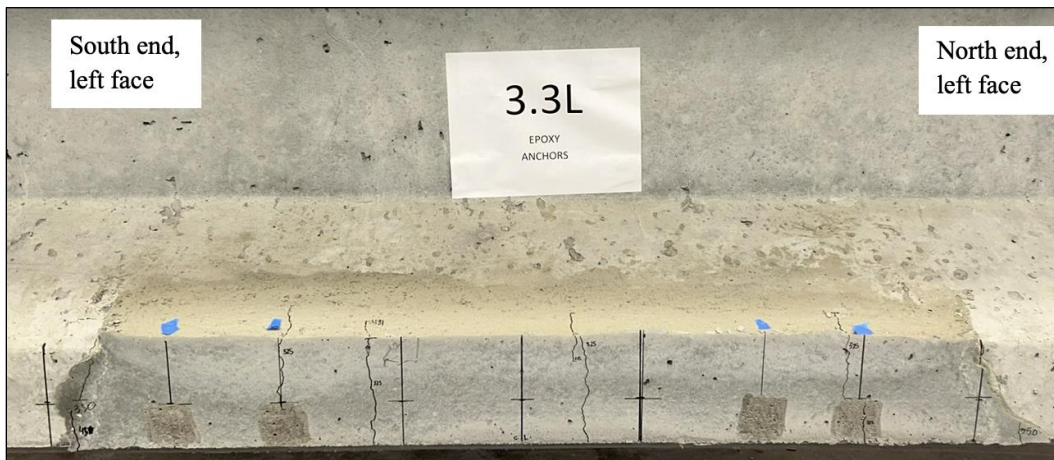
Figure 138. Photo. Test 3.1.S (repair 3.1RBF, 3.1LBF) flexural cracking on midspan repairs at 325 kip (left face of girder pictured).
