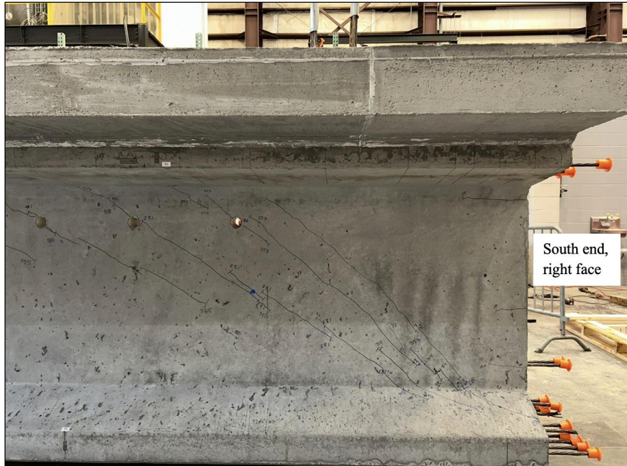
Figure 121. Photo. Test 2.2.S (repair 2.2LTF) final shear cracks on nonrepaired, original face at 424 kip (right face of girder pictured).
