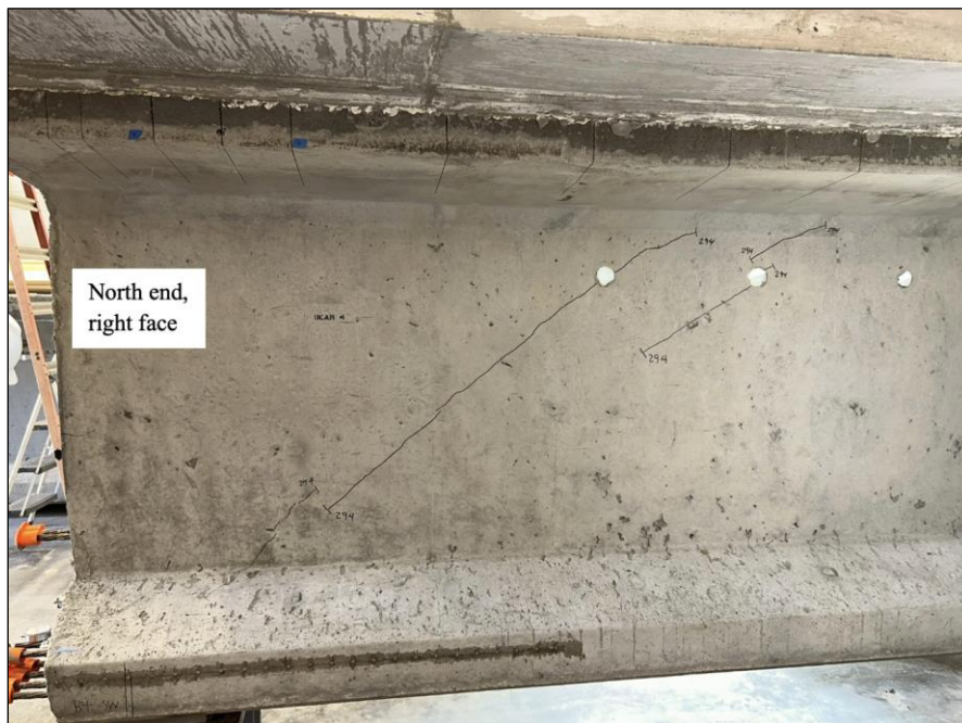
Figure 164. Photo. Test 4.1.S (repair 4.1LBZ, 4.1RTF, 4.1LTF, 4.4LTF) initial shear cracks on original, nonrepaired face at 294 kip (right face of girder pictured).
