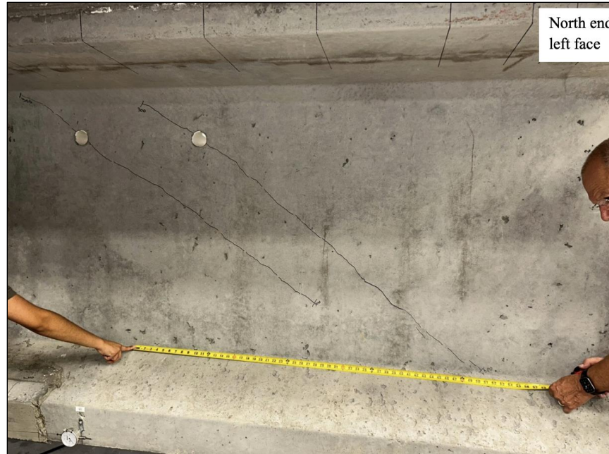
Figure 135. Photo. Test 3.1.S (repair 3.1RBF, 3.1LBF) initial shear cracks (left face of girder pictured).
