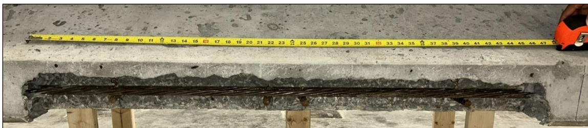
Figure 7. Bottom flange nonconformity requiring a chimney formwork for concrete replacement.
