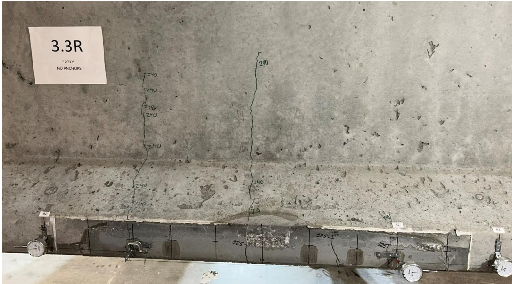
Figure 157. Photo. Test 3.3.F (repair 3.3RBF, 3.3LBF) initial flexural cracks at 240 kip (right face of girder pictured).
