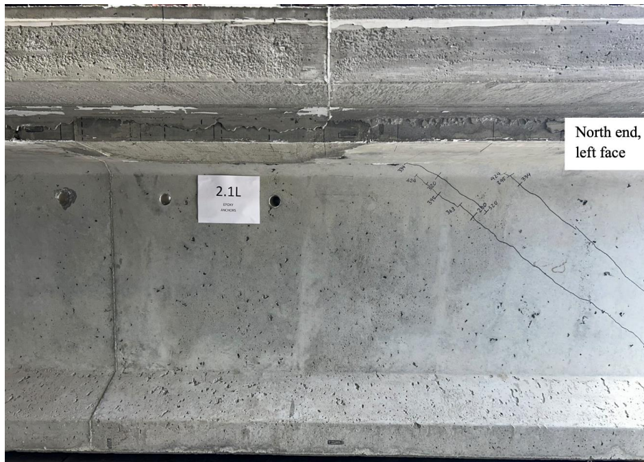
Figure 113. Photo. Test 2.1.S (repair 2.1RTF, 2.1LTF) final shear cracks not spreading to top flange repair 2.3LTF at 424 kip (left face of girder pictured).
