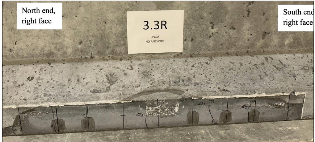
Figure 137. Photo. Test 3.1.S (repair 3.1RBF, 3.1LBF) flexural cracking on midspan repairs at 325 kip (right face of girder pictured).
