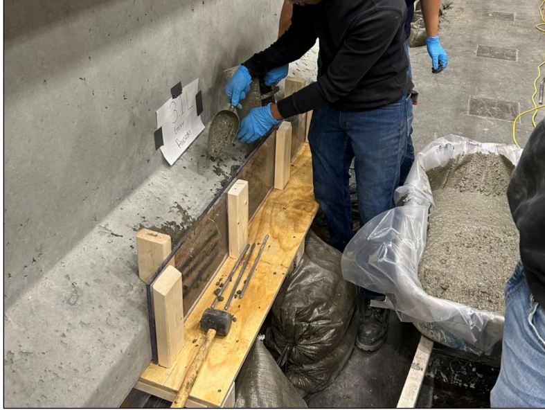
Figure 50. Photo. Placing concrete through the exposed top of a repair with polycarbonate formwork for viewing.
