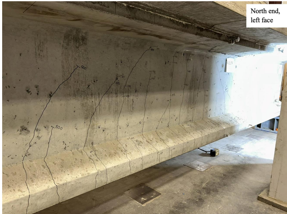
Figure 168. Photo. Test 4.1.S (repair 4.1LBZ, 4.1RTF, 4.1LTF, 4.4LTF) flexural and shear-flexural cracks around the innermost spreader beam support, not extending into repair 4.1LTF at 500 kip (left face of girder pictured).
