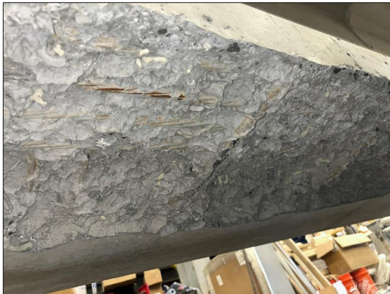
Figure 12. Bottom flange nonconformity with no exposed reinforcement.
