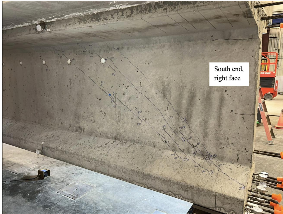
Figure 117. Photo. Test 2.2.S (repair 2.2LTF) initial shear cracks on original, nonrepaired face (right face of girder pictured).
