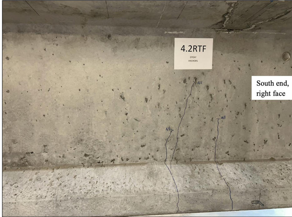
Figure 179. Photo. Test 4.2.S (repair 4.2RBZ, 4.2RTFE, 4.2RTF, 4.2LTF) initial flexural and shear-flexural cracks at 411 kip (right face of girder pictured).
