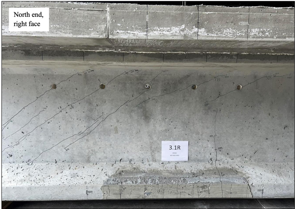
Figure 141. Photo. Test 3.1.S (repair 3.1RBF, 3.1LBF) final crack pattern at 431 kip (right face of girder pictured).
