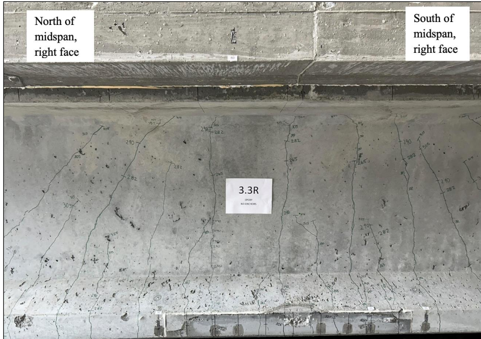
Figure 160. Photo. Test 3.3.F (repair 3.3RBF, 3.3LBF) overall crack pattern at the final load of 330 kip. Extensive flexural cracks occurred in the bottom flange repair (right face of girder pictured).
