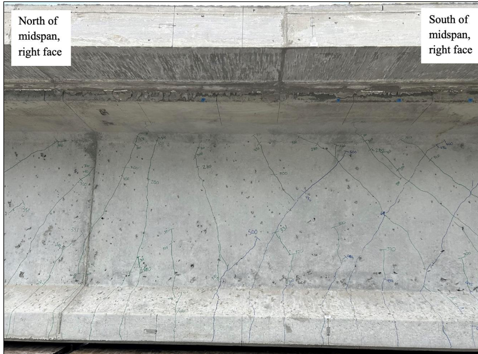
Figure 192. Photo. Test 4.3.F (repair 4.3LBF, 4.3LTF) final overall crack pattern on original, nonrepaired girder face after the final load of 331 kip (right face of girder pictured).
