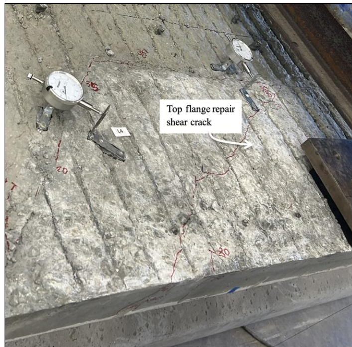
Figure 106. Photo. Test 1.4.F (repair 1.3RTF, 1.3LTF) top flange shear crack on repair 1.3LTF.
