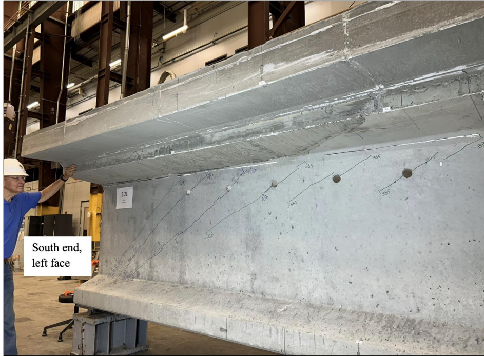
Figure 129. Photo. Test 2.3.F (repair 2.3LTF) shear cracks through tie-down holes toward the midspan of the girder at a 335-kip flexural load, repaired face with longest top flange repair of 126 in. (left face of girder pictured).
