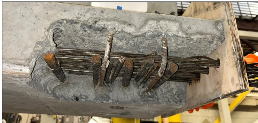
Figure 65. Photo. A nonconformity in the transfer region of Girder 1 before repair.
