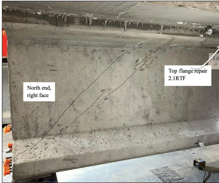
Figure 109. Photo. Test 2.1.S (repair 2.1RTF, 2.1LTF) shear cracks to the left of repair 2.1RTF (right face of girder pictured).
