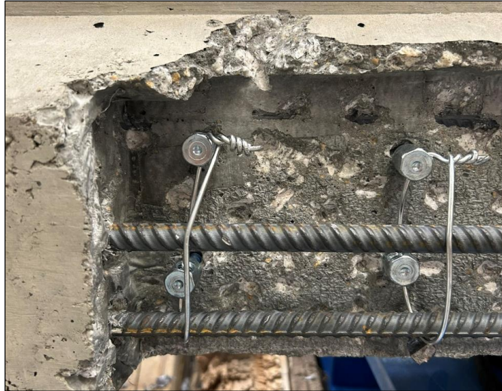
Figure 35. Photo. Practice installation of 12-gauge wire fed through the concrete anchor holes on longitudinal reinforcement.
