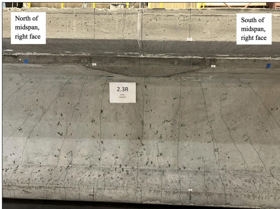
Figure 130. Photo. Test 2.3.F (repair 2.3LTF) final flexural and shear-flexural cracks on repaired face at 341 kip. Cracks did not extend into top flange repair 2.3RTF (right face of girder pictured).
