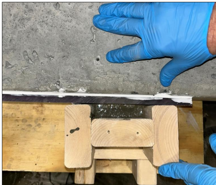
Figure 52. Photo. SCC flowing out of the air vent and through the drilled hole, indicating complete concrete replacement in the repair.
