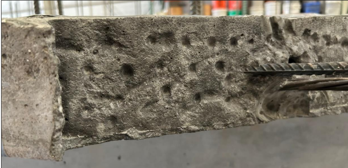
Figure 3. Top flange 0.25-in. amplitude chipped surface.
