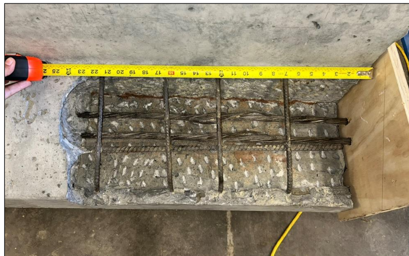
Figure 67. Photo. A nonconformity in the transfer region of Girder 4 before repair.
