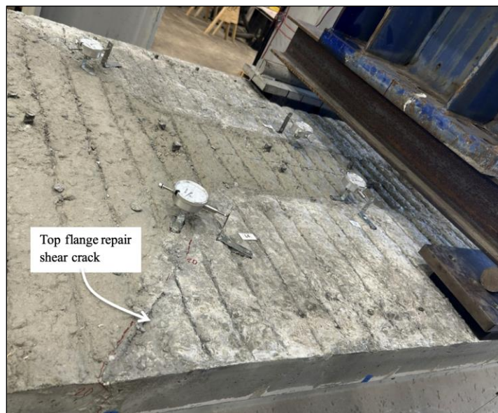
Figure 105. Photo. Test 1.4.F (repair 1.3RTF, 1.3LTF) top flange shear cracks at 20 kip (left face of girder pictured).
