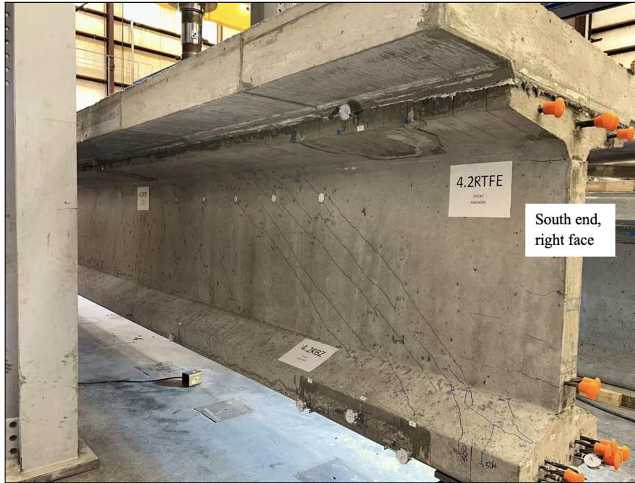
Figure 181. Photo. Test 4.2.S (repair 4.2RBZ, 4.2RTFE, 4.2RTF, 4.2LTF) final shear cracks on top and bottom flange repaired face at 500 kip (right face of girder pictured).
