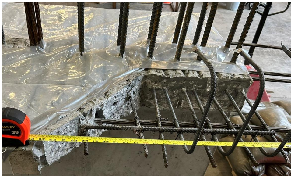
Figure 2. Top flange nonconformity located at the end of the girder.
