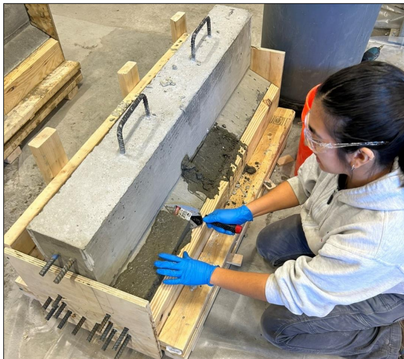
Figure 38. Photo. Finishing the SCC repair surface with a trowel for Mini Girder 1.
