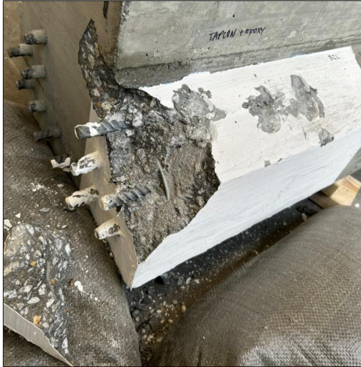
Figure 42. Photo. Intense sledgehammering removed corner concrete and demonstrated good consolidation of concrete around the reinforcement and 12-gauge wires.
