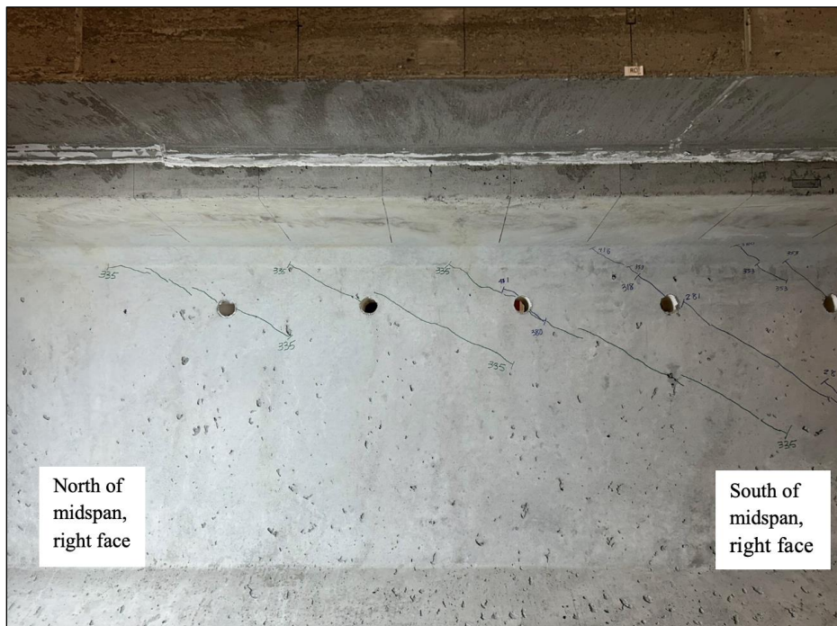
Figure 128. Photo. Test 2.3.F (repair 2.3LTF) shear cracks through tie-down transport holes toward the midspan of the girder at a 335-kip flexural load, nonrepaired, original face (right face of girder pictured).
