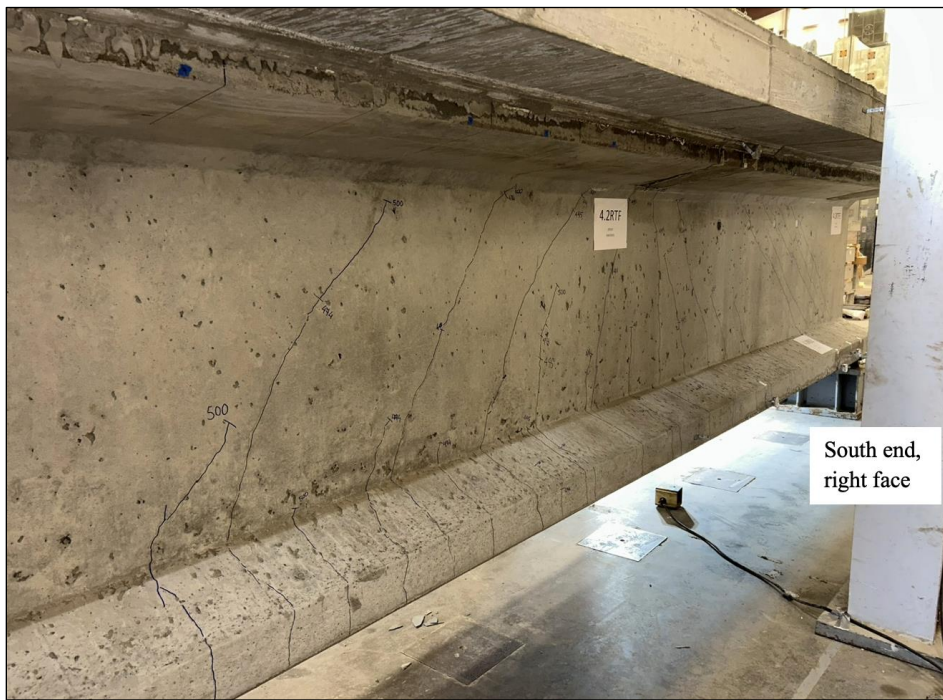
Figure 183. Photo. Test 4.2.S (repair 4.2RBZ, 4.2RTFE, 4.2RTF, 4.2LTF) flexural and shear-flexural cracks around the innermost spreader beam support, extending slightly into repair 4.2RTF at 500 kip (right face of girder pictured).
