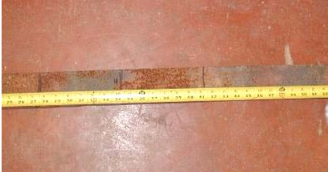
Figure 3.7 Heated Areas in Blue on Eyebar 2
