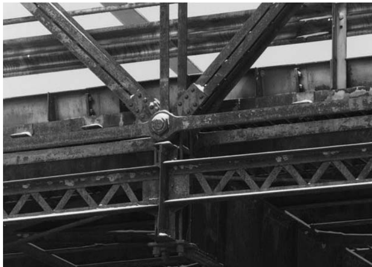
Figure 5.4 Typical Eye Pin Connection (Walnut Street Bridge, Spanning Susquehanna River at Walnut Street, Dauphin County, PA - Historic American Buildings Survey/Historic American Engineering Record)
