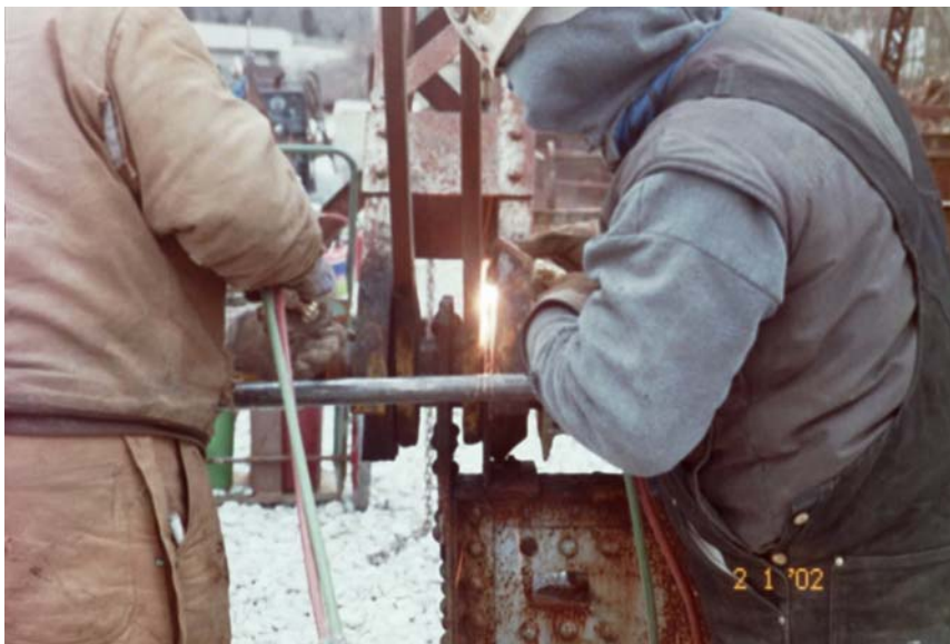
Figure 5.6 Using Heat to Help Remove a Pin During a Rehabilitation of a Bridge In Plainfield, IN.
