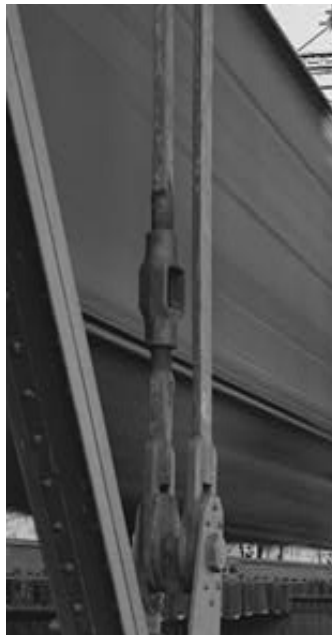
Figure 5.12 Typical Turnbuckle found in and Existing Wrought Iron Bridge (Penn. Railroad, Selinsgrove Bridge, Spanning Susquehanna River, Snyder County, PA - Historic American Buildings Survey/Historic American Engineering Record)
