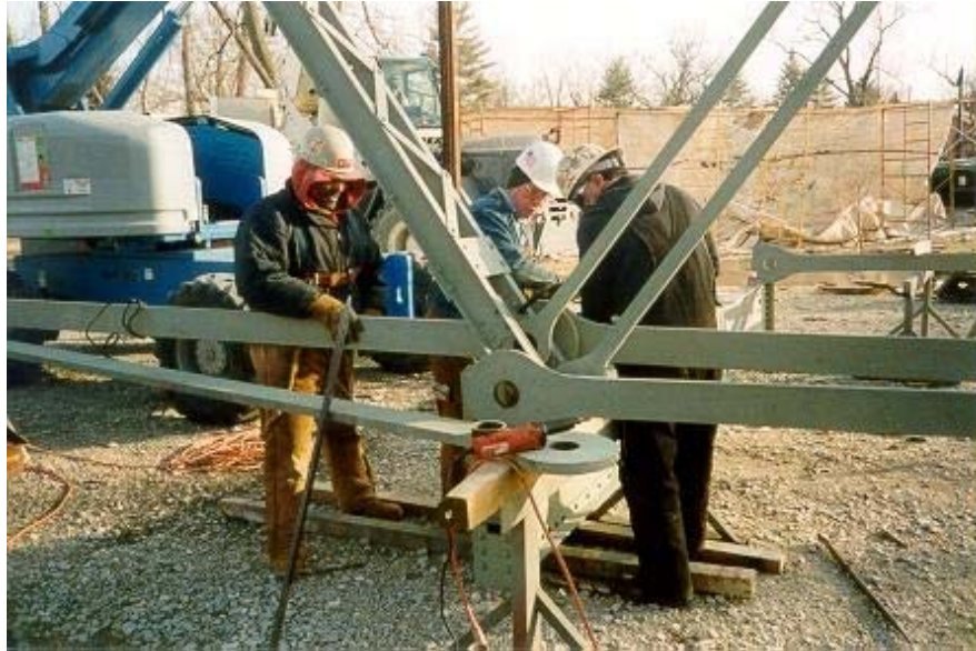
Figure 5.11 Reassembling a Pin Connection After Members Have Been Sand Blasted and Repainted During A Rehabilitation of a Bridge in Plainfield, IN
