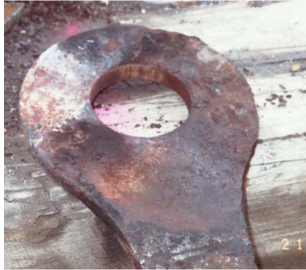
Figure 5.9 Heavy Corrosion in an Eyebar End Connection
