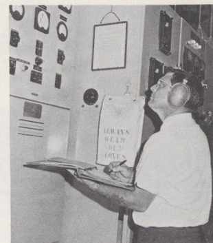
Building Manager Ed Dobb keeps a regular record of engine generator performance at the world's busiest air traffic control center. Housed in a separate building, the generators create enough noise to require technicians to wear protective ear-covers.
