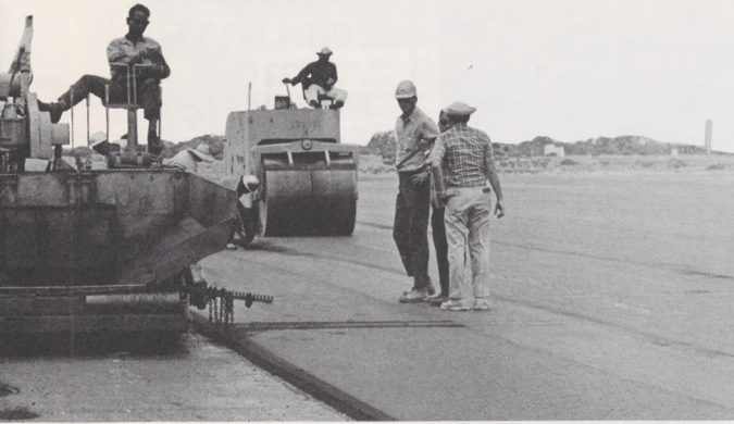
dem roller were used to lay asphaltic concrete runways at Wake Island Airport.
