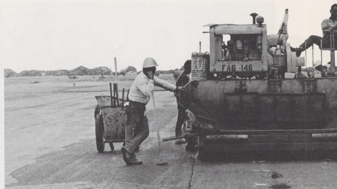
Barber Greene bituminous asphalt spreader and ten-ton tandem roller were used for runway construction.
