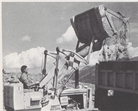
Loading a ten-wheeler is Hal Wright, heavy equipment operator, at the controls of a skid-shovel. Photo was taken at Francis Peak near Salt Lake City, near one of the agency's long-range radar sites.
