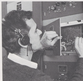
Electrical circuits in the Tweed-New Haven Tower are checked by Electronics Technician John Dorey from the Boston Area Office.
