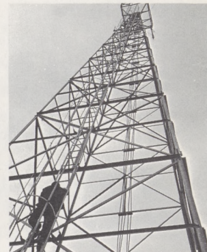
An FAA maintenance man (electronic technician) must climb tall towers periodically to keep NAVAIDS going properly. This one rises 108 feet above the summit of English Mountain near Knoxville.
