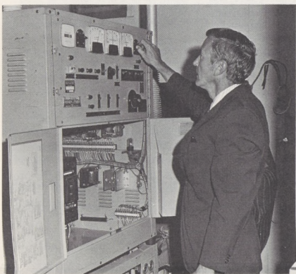
Sometimes a technician can read a half-dozen meters and flick some switches to put electronic equipment back into operation quickly. Here Herman E. Williams, Knoxville Sector Chief, checks equipment in the Snowbird VOR.
