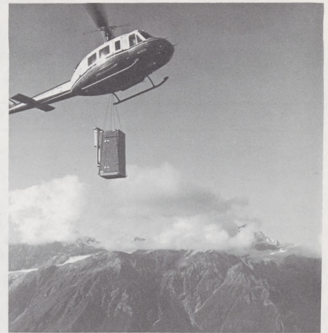
Everything had to be transported by helicopter to the rocky shelves of Lake Clark Pass. Here a Bell 205A-1 moves a 1,500-pound shelter component to Site 1.
