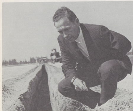
Every detail, large and small—such as this lighting cable installation at North Perry Airport—receives close scrutiny.
