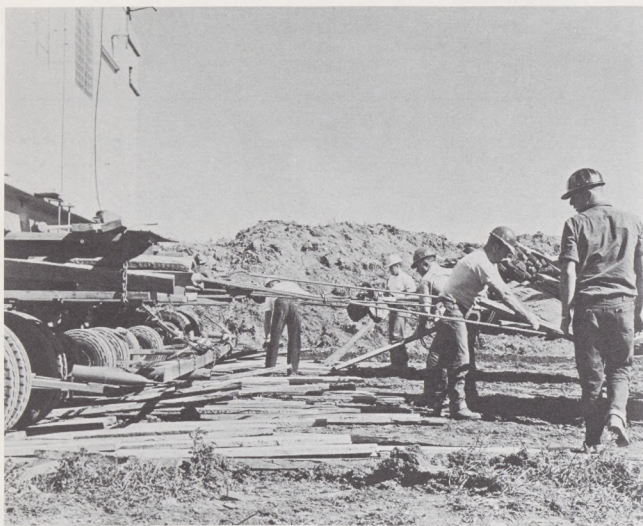
Members of the Berg and Henn Company's crew lay the landing mat of two-inch elm planks upon which the load was moved.
