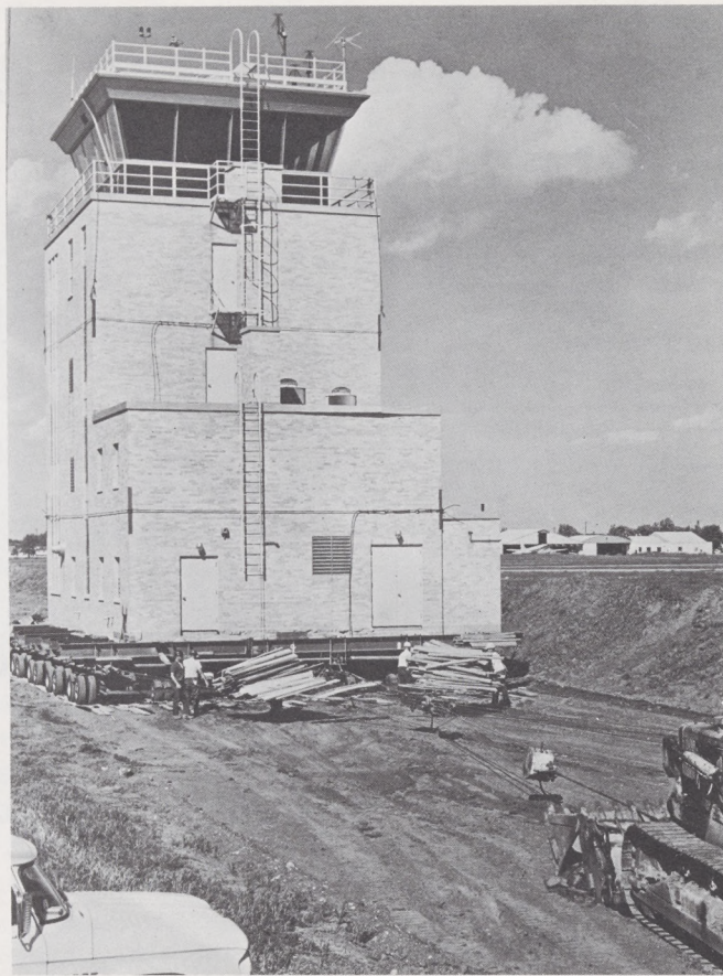
Tower on the move—note earth pile on the right which resulted from grading the haul road. Moving contract called for restoring land configuration when move was finished.
