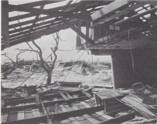
Wooden structures, mostly owned by Pan American Airways, didn't fare too well. Heaviest damage to family housing was to those located along the beach. Families living there lost most of their personal possessions when rain, winds and high waves demolished their homes.
